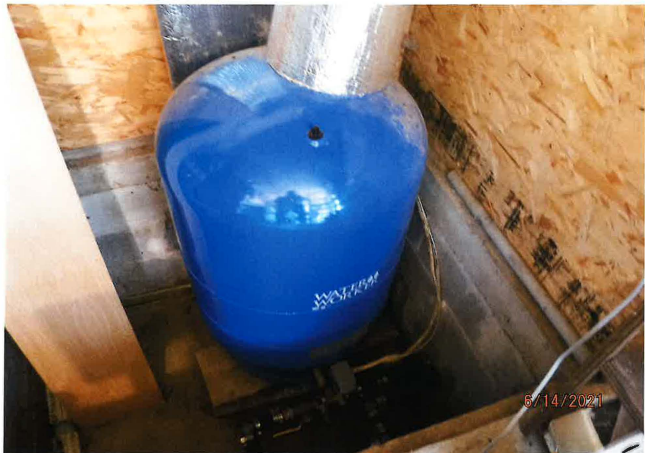
DIVERSION WORKS – PIPE FROM WELL DIRECT TO PRESSURE TANK
