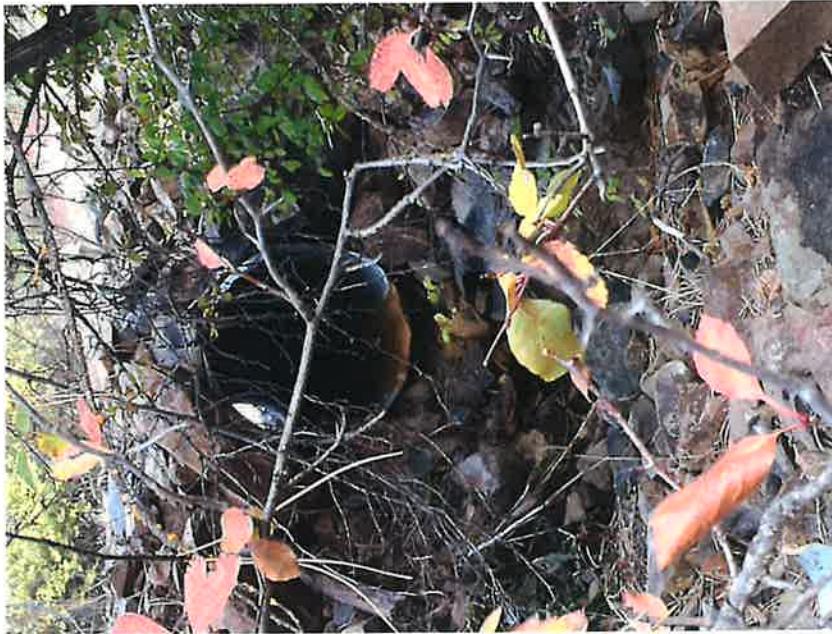
Image 1. The culvert that conveys flow from the unnamed stream to the Bear Community Ditch. This view is looking at heading 340 degrees (upstream view).
