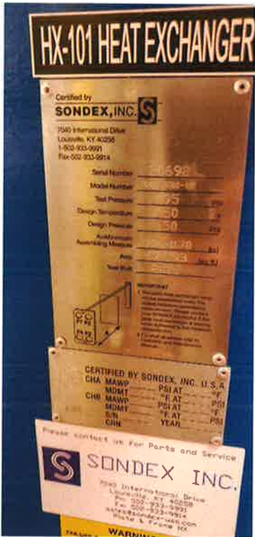
Figure 4: Data Plates on Heat Exchanger
