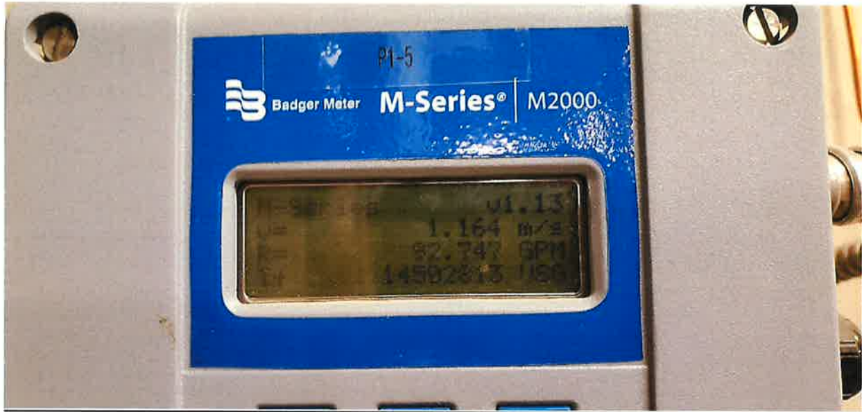
Figure 1: School's in-line magnetic meter (note the gallons per minute)
