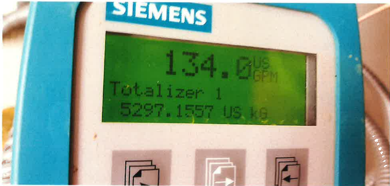
Figure 1: Readout on installed meter during measurement
