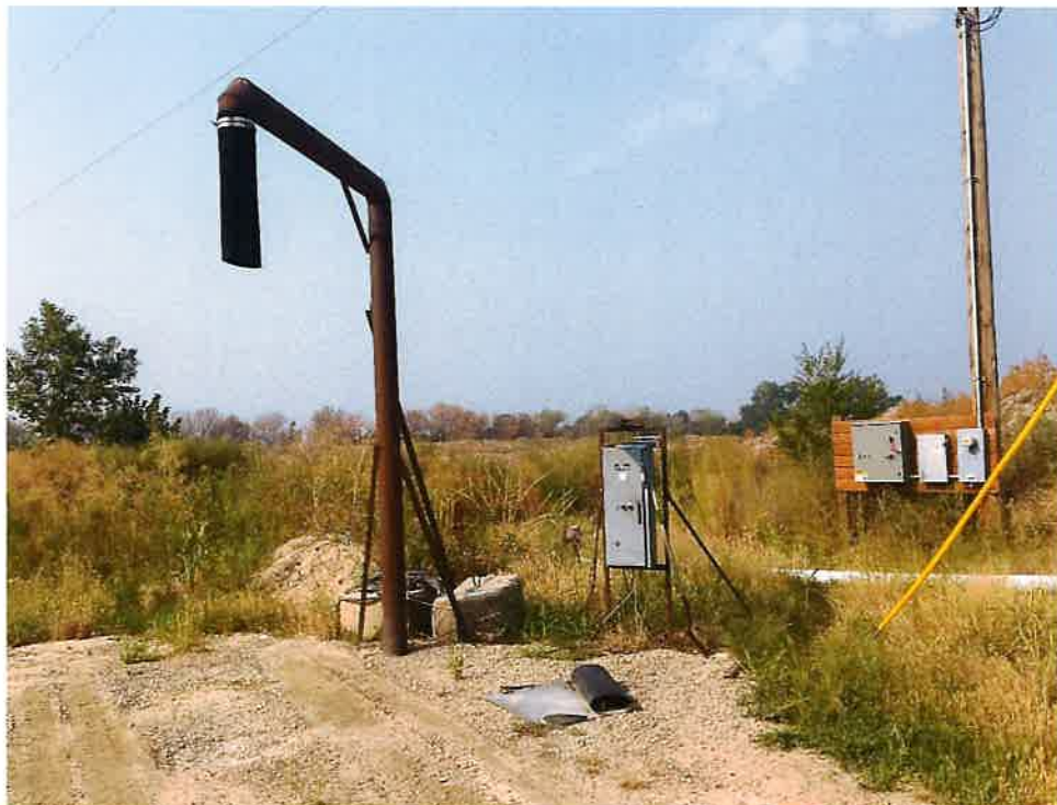
Figure 6: Truck fill station
