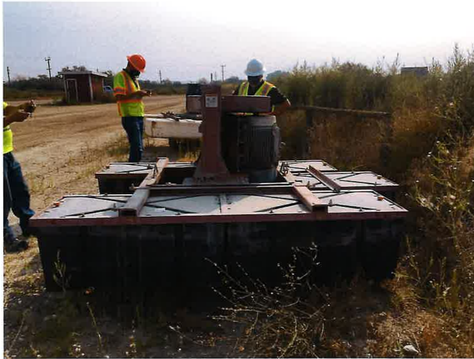
Figure 7: One of the floating Fisher pumps that can be used on the property.
