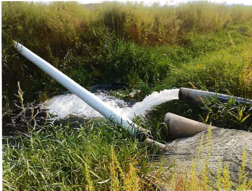
Figure 4: Photo of the discharge pipe
