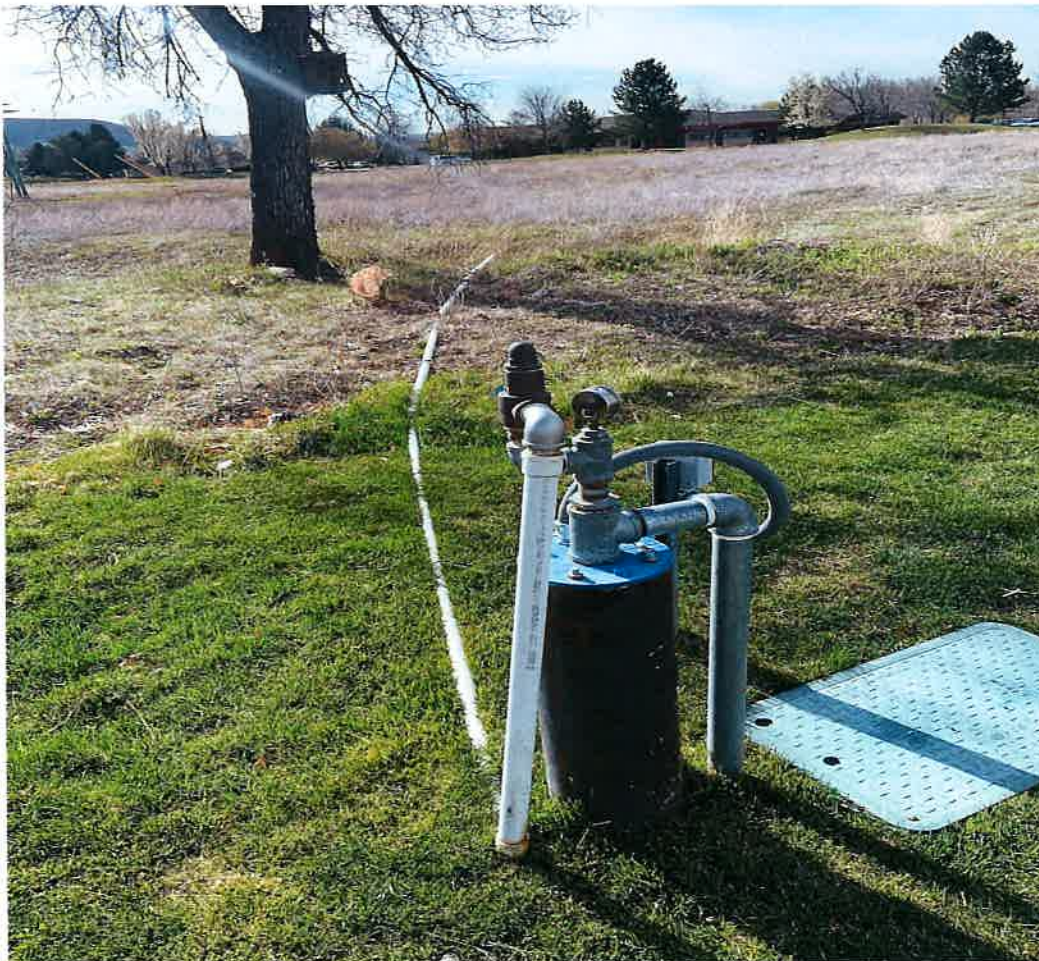
Fig. 2 – The well overflow/back pressure goes to a ditch that appears to flow into the Boise River.
