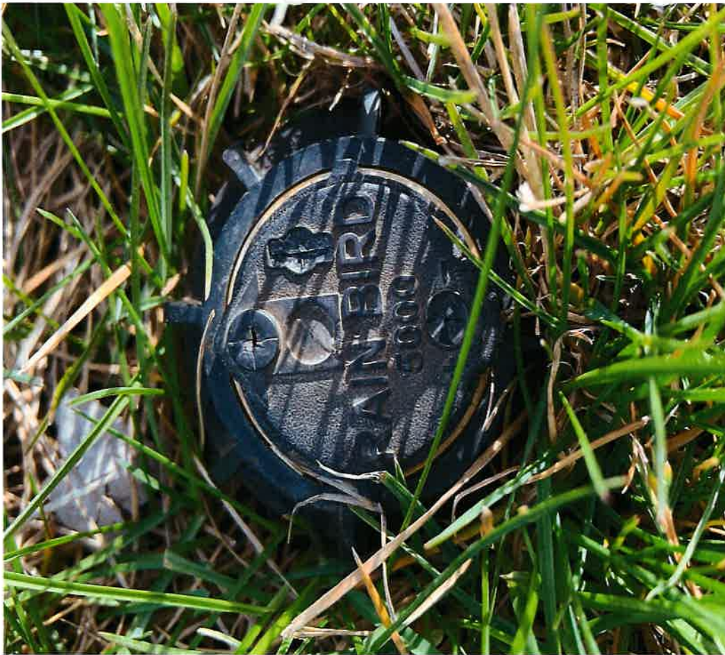
Fig. 5 – Pop-up sprinklers for the sports field are Rainbird 5000. There are approx. 70 sprinklers for the field.
