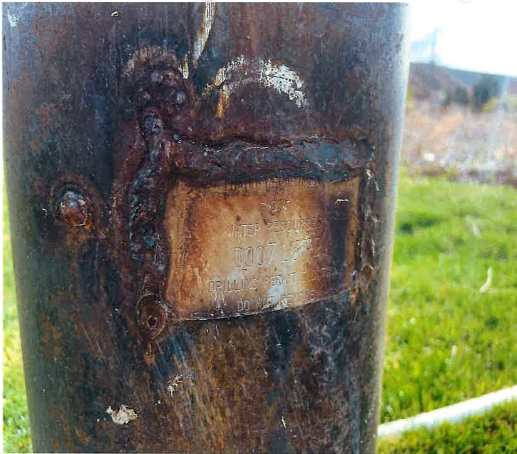
Fig. 3 – Well tag ID #D0071679 has an 8" casing from 2-67 ft bsl, and contains a 1.5 hp pump.
