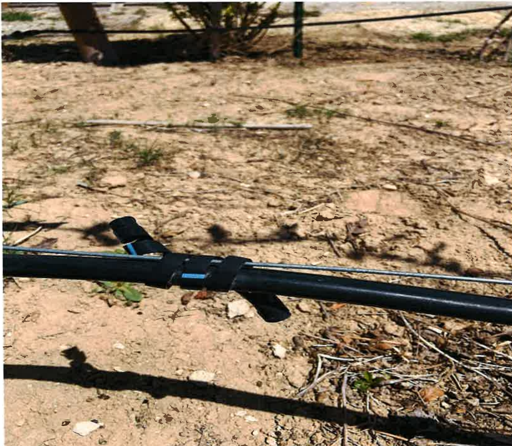
Fig. 10 – A close up view of the 1" poly lines that deliver well water to the vineyard. The spiraled material causes the water to drip into the soil in a set location.
