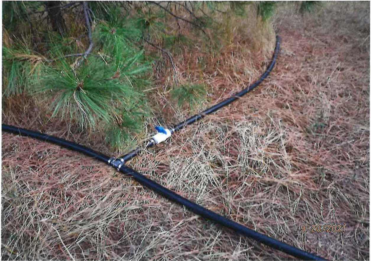
IRRIGATION FROM STORAGE POU – SOUTH POND MAIN TRUNK POLY PIPE WITH TEE JUNCTION PIPE
