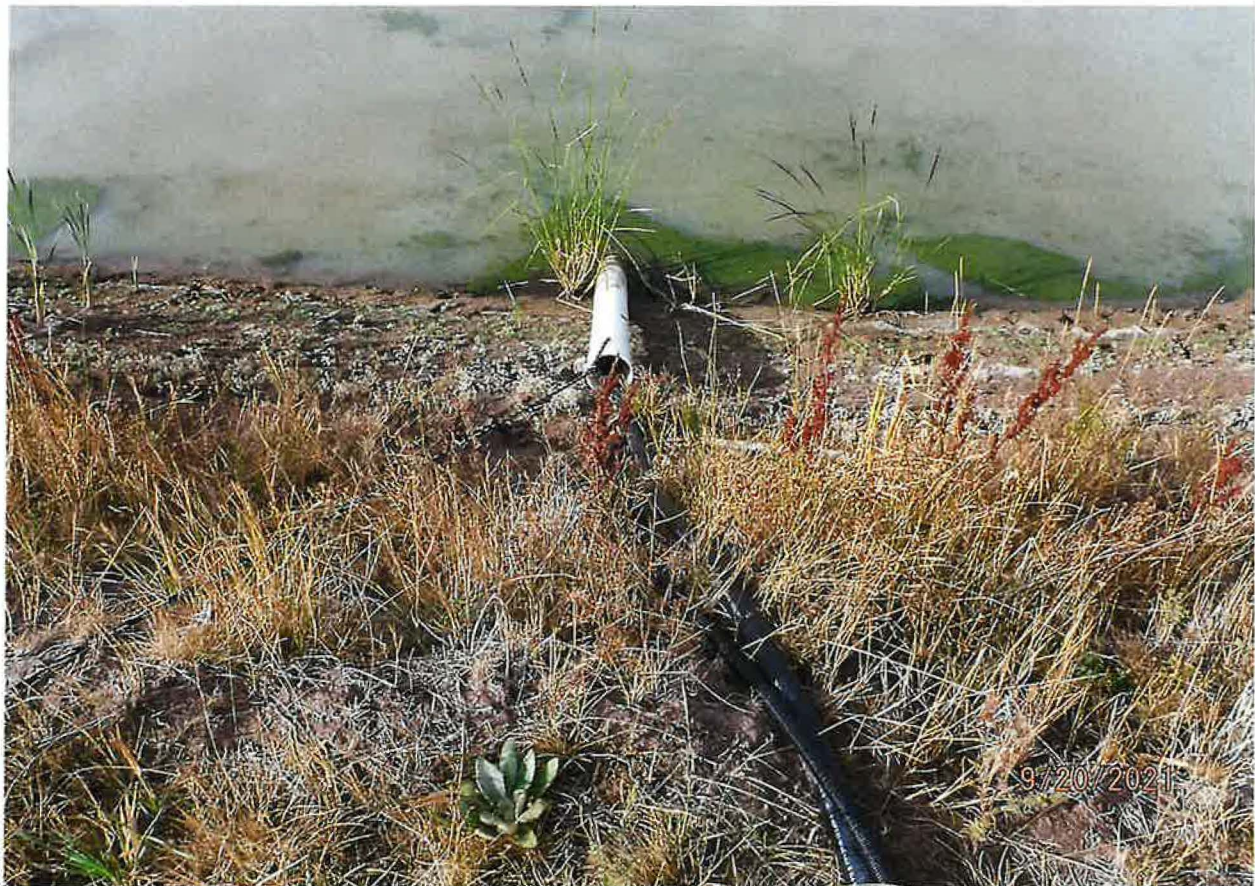
SOUTHERN POND – 1 HP TRANSFER PUMP ROUTES WATER TO NORTHERN POND FOR USE
