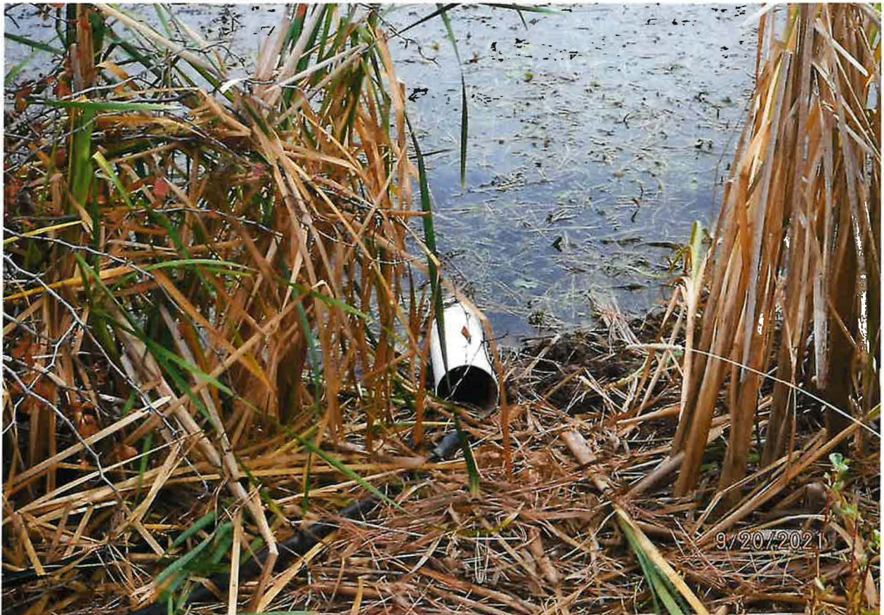
NORTHERN POND ½ HP SOLAR POWERED PUMP USED FOR IRRIGATION FROM STORAGE USE
