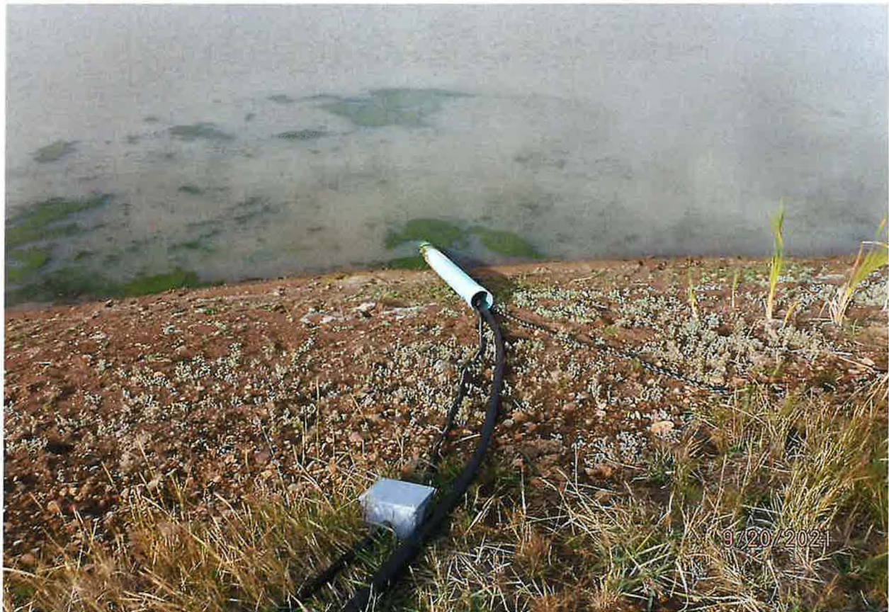
SOUTHERN POND – 1 HP SOLAR POWERED PUMP FOR IRRIGATION FROM STORAGE USE
