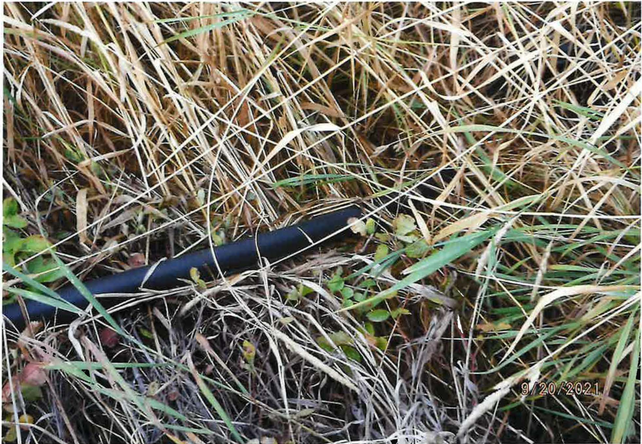
1 INCH POLY PIPE SERVICE PIPE TO TRANSFER WATER FROM SOUTH TO NORTH POND
