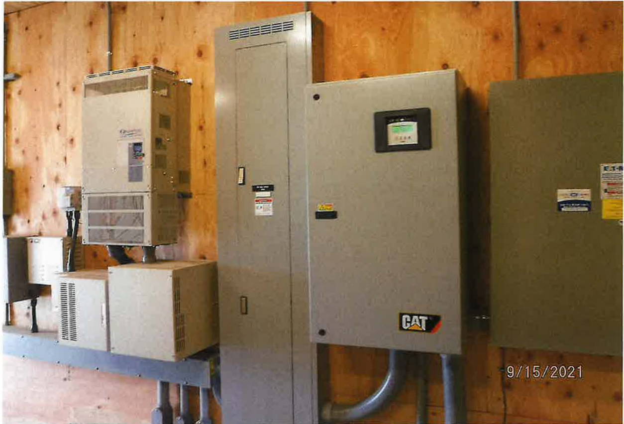
ELETRONIC CONTROL PANELS
