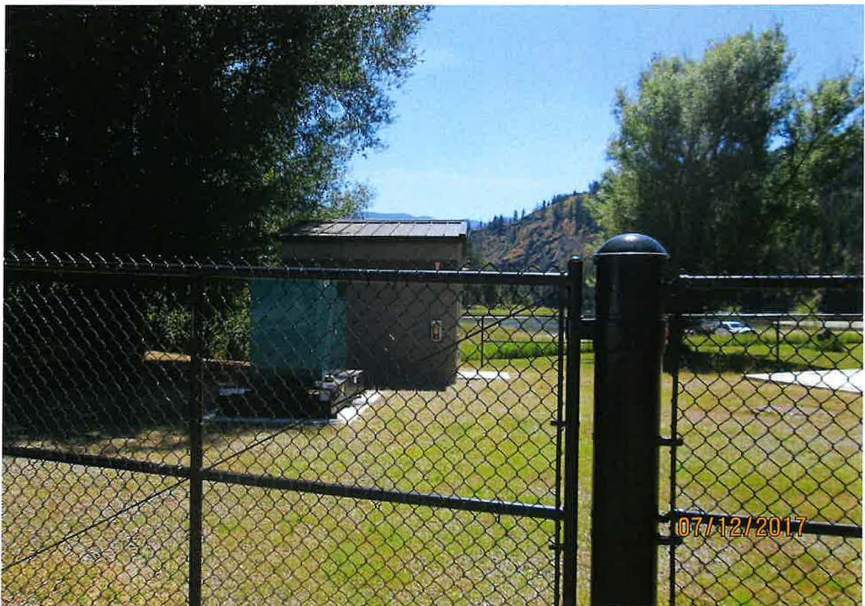
KOOTENAI RIVER CONVEYANCE SYSTEM PUMP STATION
