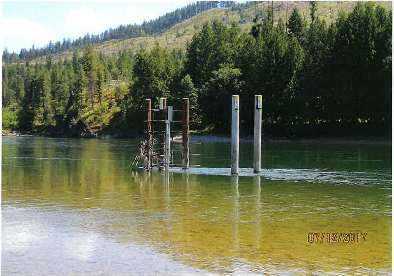
POD – KOOTENAI RIVER INTAKE WORKS
