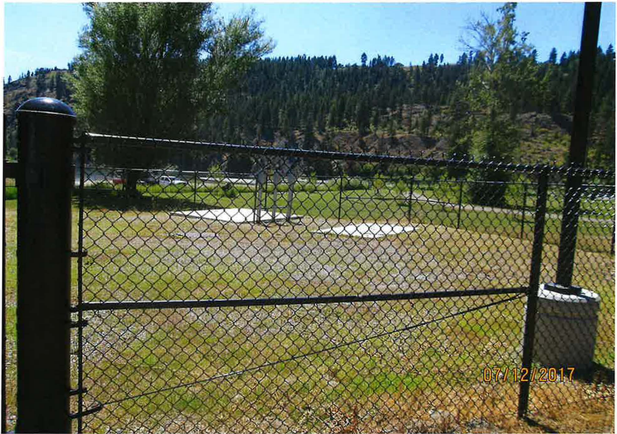
KOOTENAI RIVER CONVEYANCE SYSTEM PUMP STATION PIPE VAULT(S)
