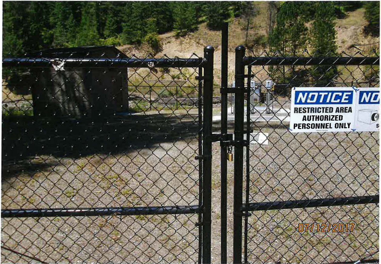
MOYIE RIVER CONVEYANCE SYSTEM PUMP STATION
