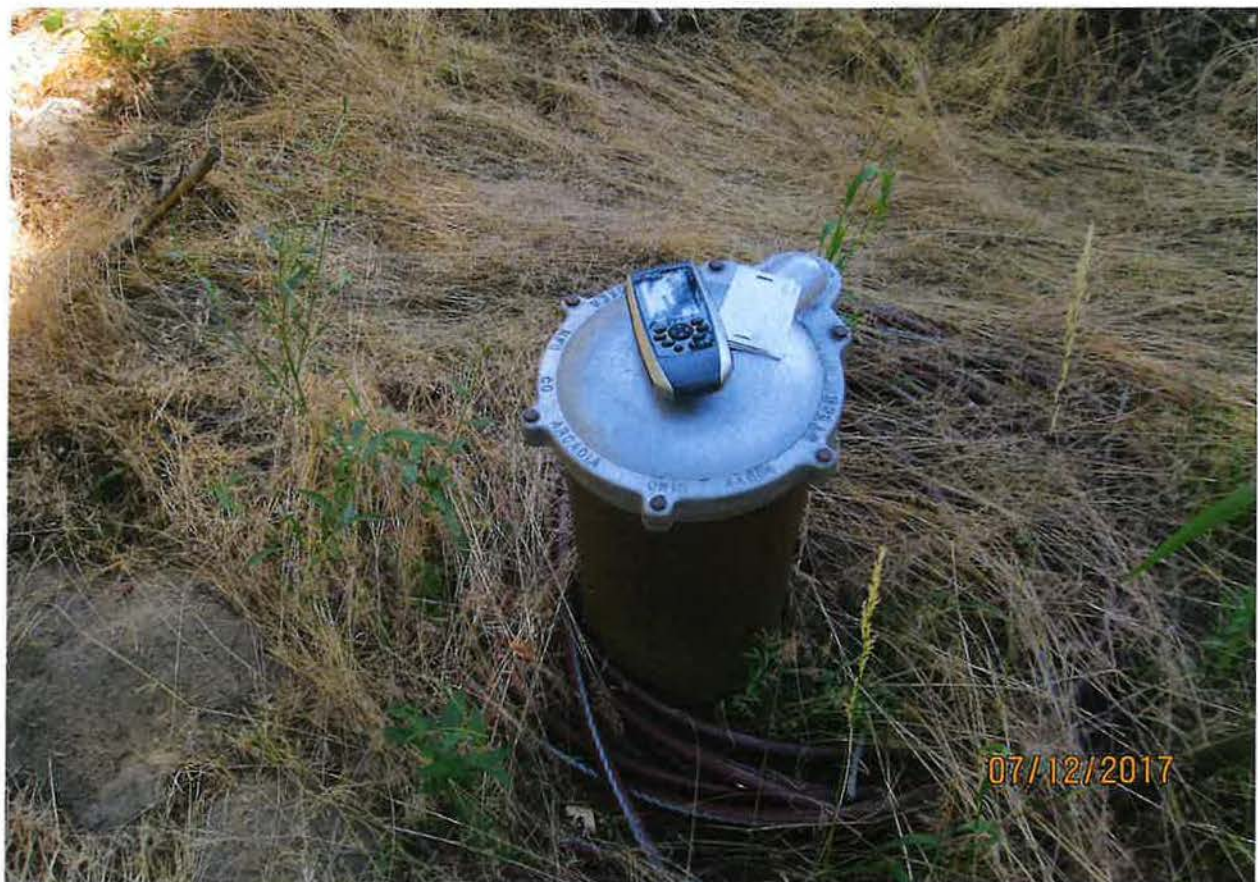
POD - WELL (98-90-N-18-000)
