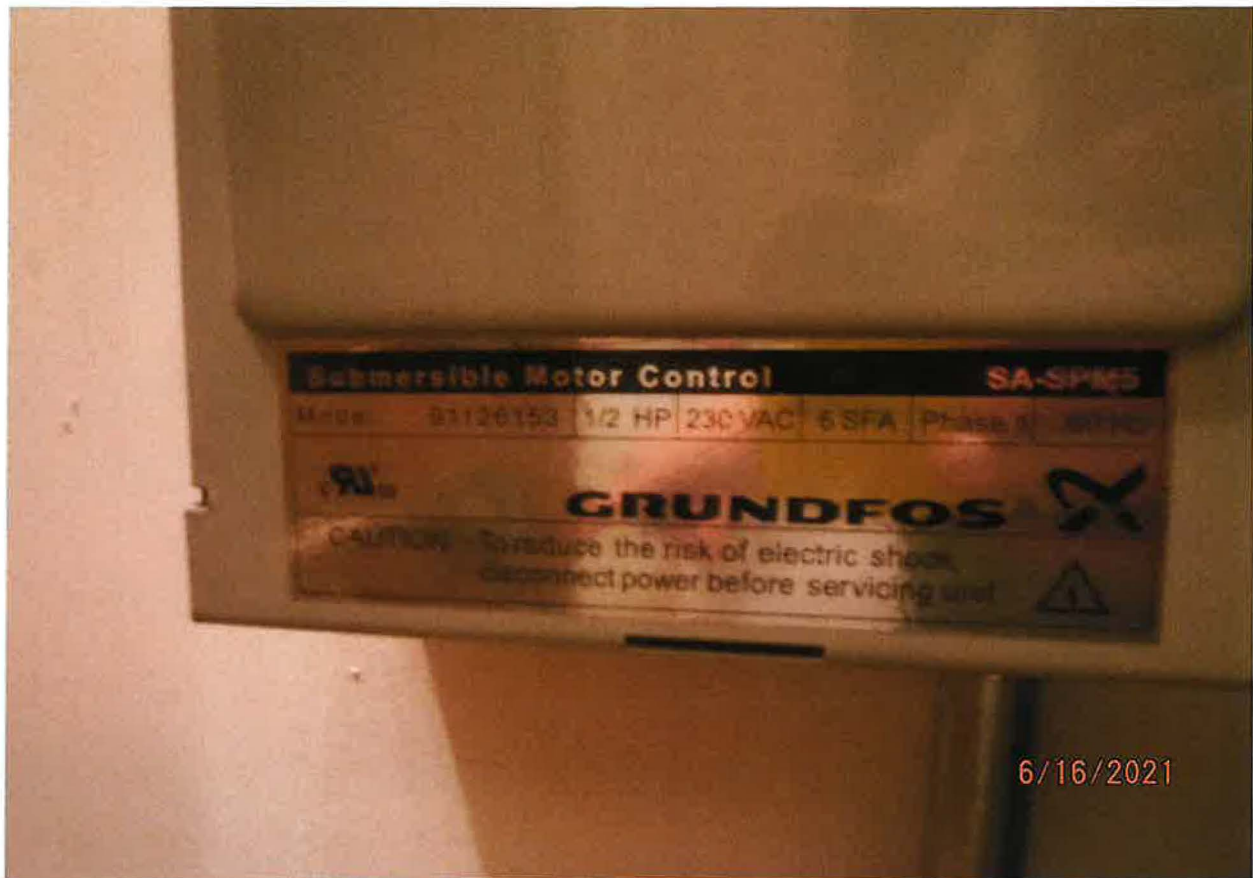
GRUNDFOS 1/2 HP SUBMERSIBLE PUMP INSTALLED IN WELL
