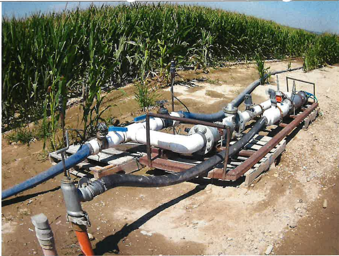
Figure 13. Manifold for drip line supply and sediment filters.
