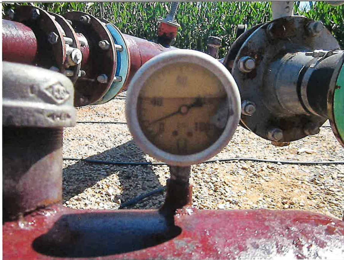
Figure 6. Pressure gage located between well and booster pump.
