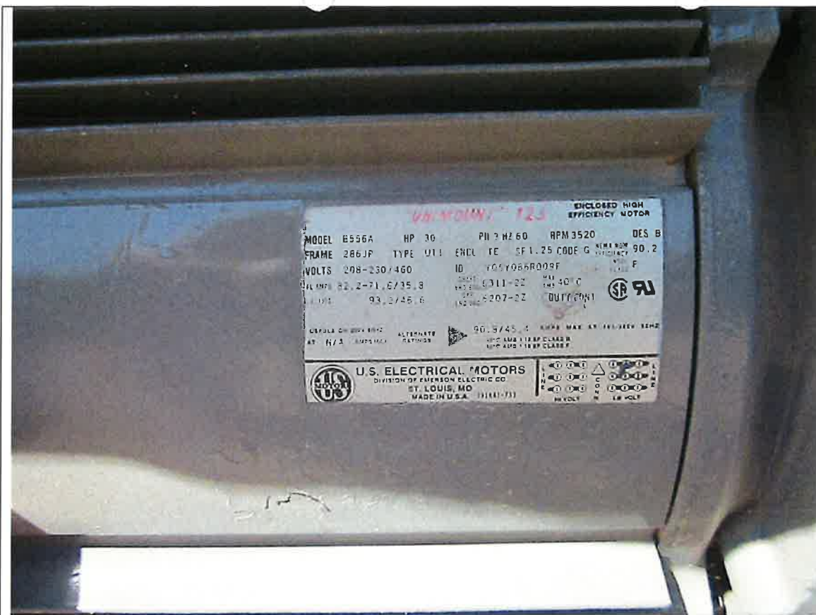
Figure 3. Tag on side of 30 hp booster pump.
