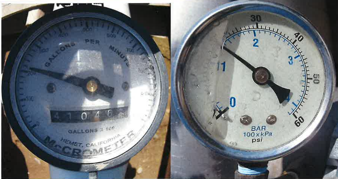
Figure 14. McCrometer flow meter on manifold showing 200 gpm at 20 psi.
