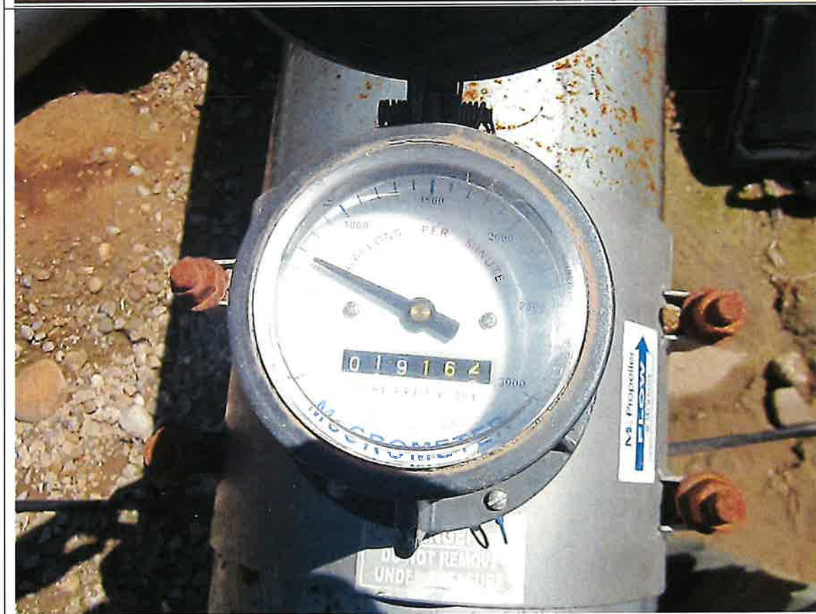
Figure 8. McCrometer flow meter reading between 675 and 700 gpm.
