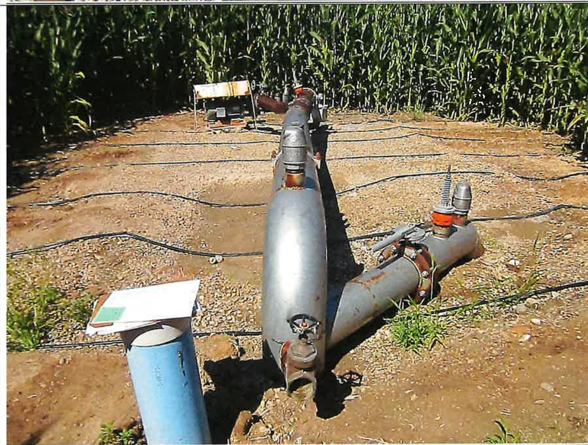
Figure 2. Pipe configuration with diagonal pipe going toward pivot and straight pipe going toward 63-33744 place of use.
