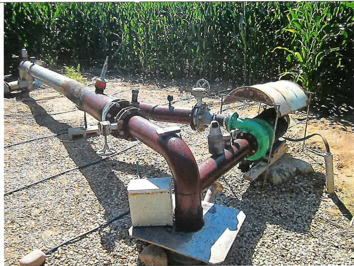
Figure 1. Well pump configuration with 30 hp booster pump.
