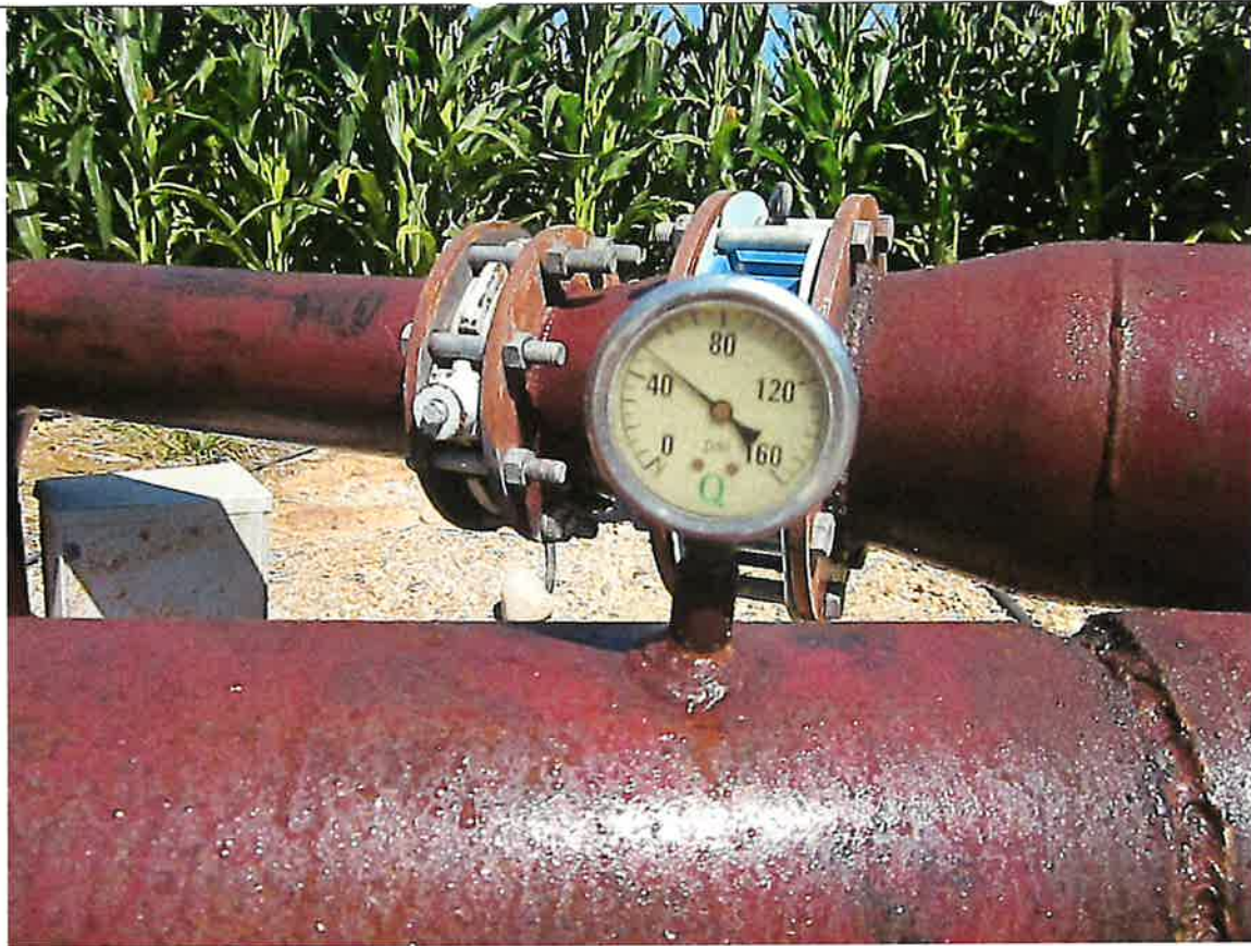
Figure 5. Pressure gage on pipe from booster pump reading about 50 psi.
