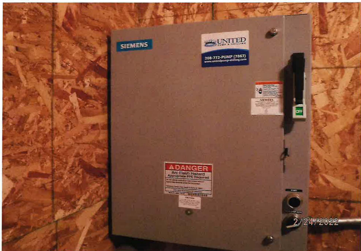
PUMP CONTROL PANEL – 20 HP PUMP/MOTOR INSTALLED, VERIFIED SEE ATTACHED PUMP INSTALL DOCUMENT
