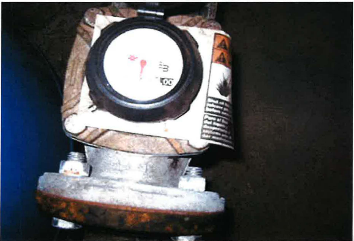
YEAR 2015 PHOTO – FLOW MEASUREMENT TAKEN FROM FLOWMETER USING WITH SYSTEM OPERATING AT MAX CAPACITY
