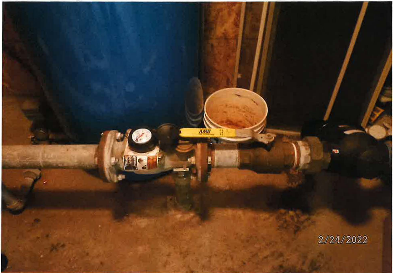
FLOWMETER INSTALLED ON WATER SYSTEM
