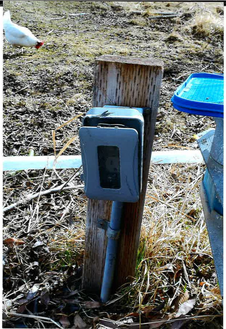
Exhibit #1-A Electric Box
