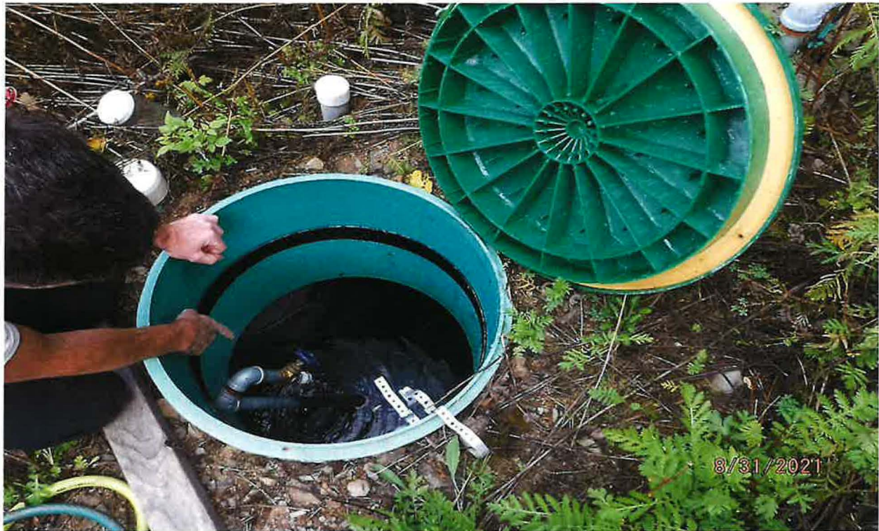
SPRING WATER ROUTED FROM POD TO 1 ST 2500 GAL STORAGE TANK (SAME DIVERTING WORKS & WATER SYSTEM INFRASTRUCTURE AS WR 96-9615)
