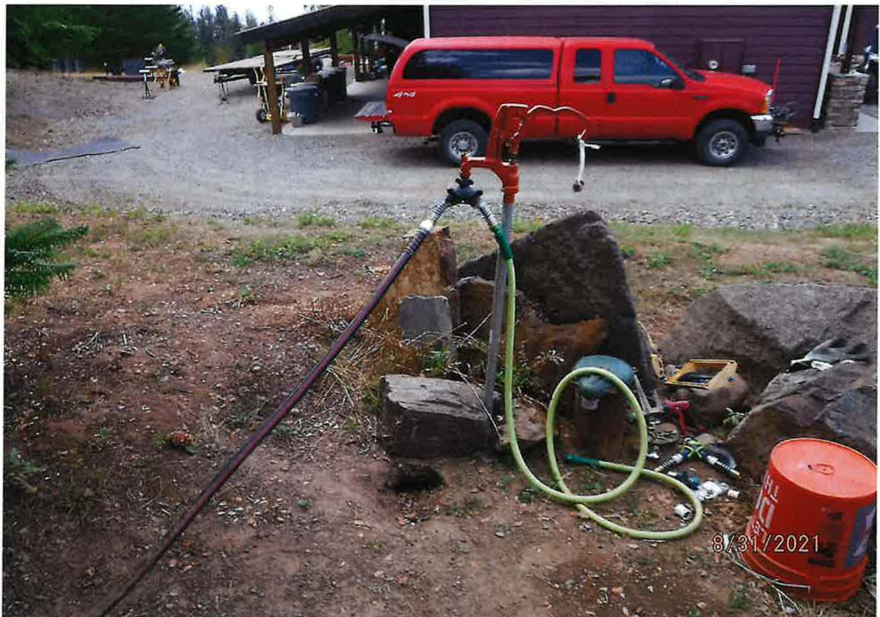
FROST FREE HYDRANT AND HOSE FROM LOWER STORAGE TANK – PROVIDES WATER TO IRRIGATION POU
