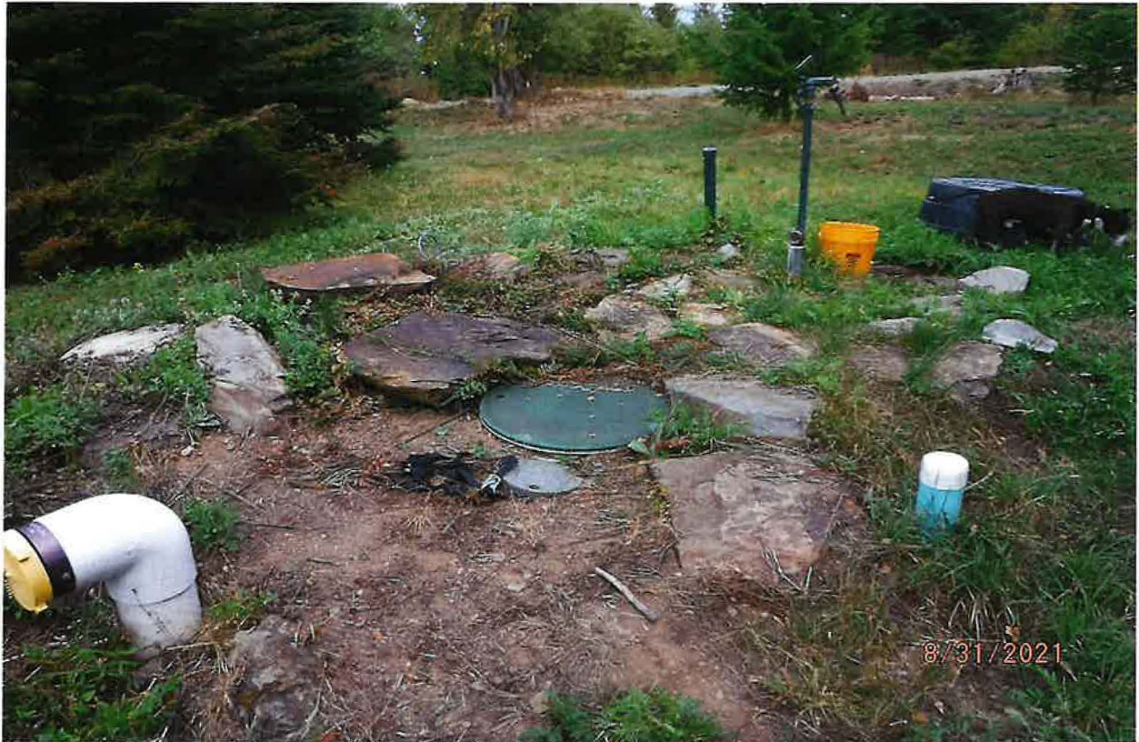
2 ND (LOWER ELEVATION) 2,500 GAL STORAGE TANK LOCATED IN LOT 2, EUEREKA HEIGHTS SUBDIVISION
