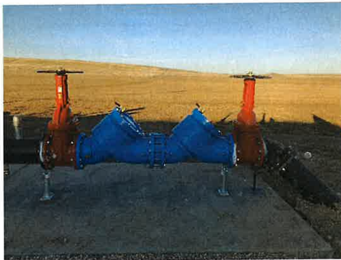
Figure 2. Backflow Preventer for Water Flowing North
