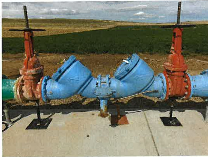
Figure 1. Backflow Preventer for Water Flowing South.
