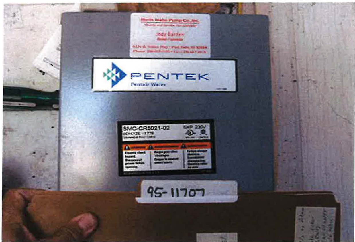
5 HP PENTEK PUMP MOTOR INSTALLED
