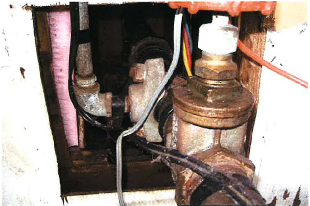
POD – WELL 95-73-N-79; LOCATED IN CRAWLSPACE OF PUMP HOUSE
