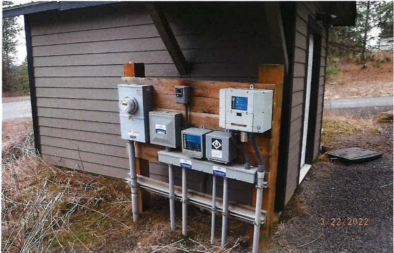
DIVERTING WORKS PUMP HOUSE, LOCATED WITH PARCEL No. RP046900010160
