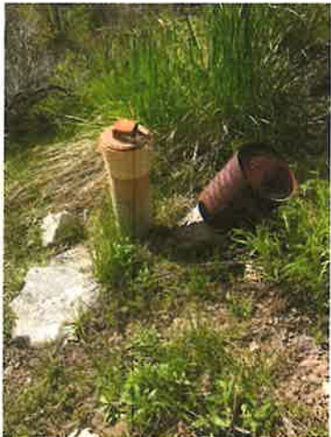
COFFEE CAN MARKER REMOVED TO EXPOSE CAPPED VALVE ACCESS TUBE
