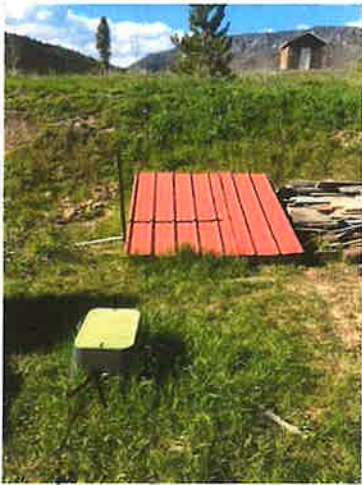
HOUSING TO PROTECT SHUT OFF VALVE TO LOWER ALTITUDE USAGE POINT
