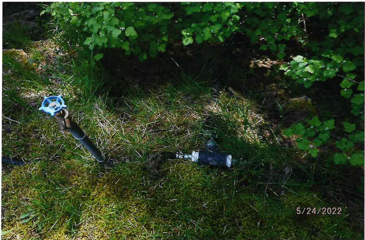
MAIN IRRIGATION LINE TO ¾ INCH POLY PIPE SPLITTER THAT TIES TO 5EA TOTAL SPRINKLER RISER PIPES WITH HOSE BIB ATTACHMENTS.
