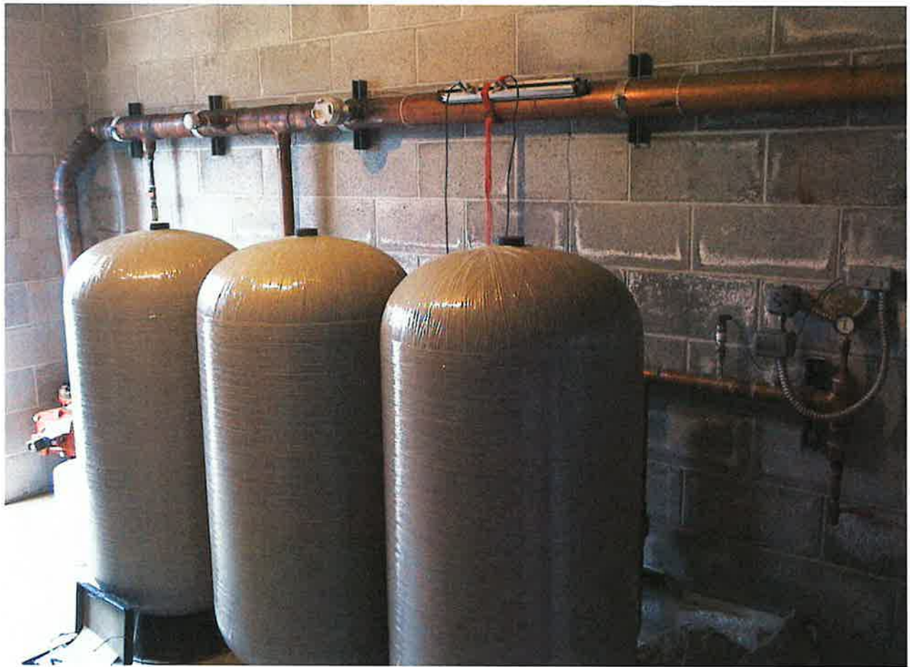
Storage tanks, facing southwest. Ultrasonic flow meter sensor attached to pipe above tanks.
