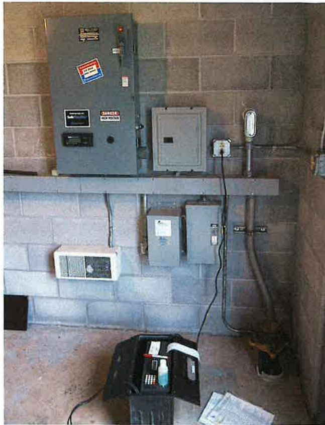
Inside well house, flow meter at bottom, facing northeast.
