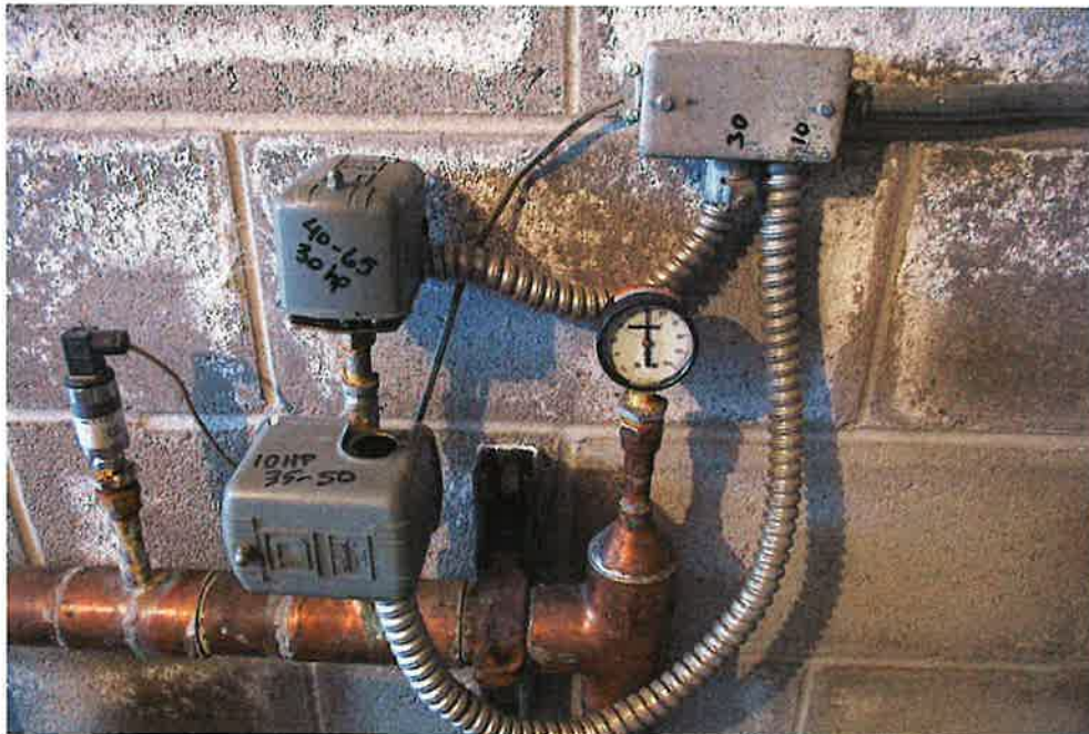
Pressure gage, reading 50 psi during measurement, and wiring with junction boxes indicated horsepower and pressure range for each well.
