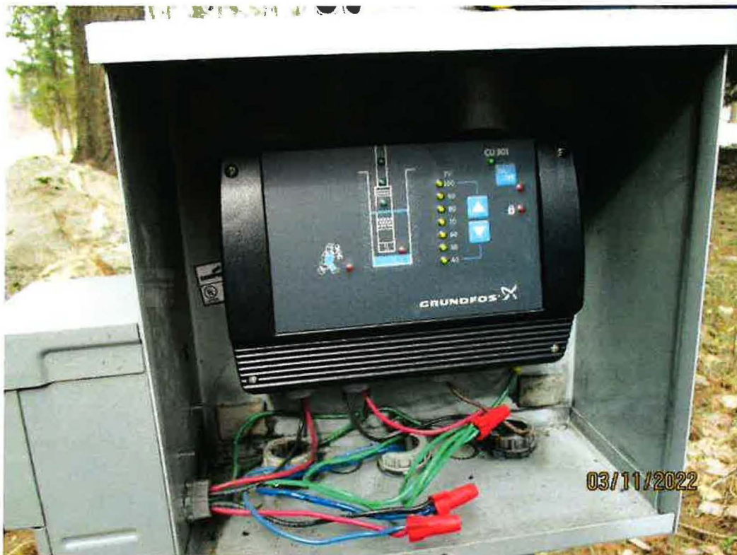
Pump Controller on Existing Well on RP56N05W297251A
