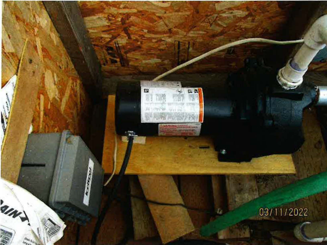
RP56N05W297251A Existing SW 1-1/2 HP Pump – used for irrigation
