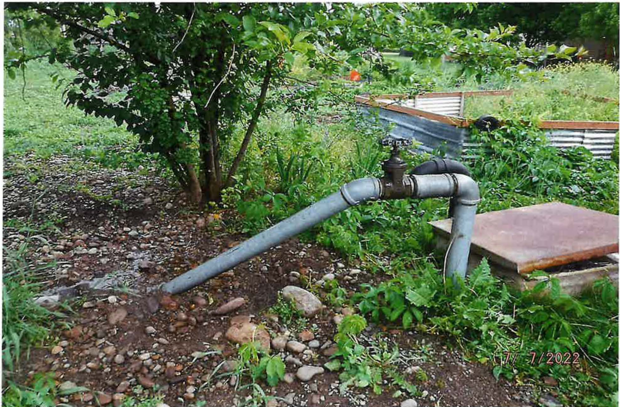
MAIN IRRIGATION SYSTEM TRUNK LINE ROUTES FROM VAULT TO HAY FIELDS ON WESTERN EXTENT OF PARCEL
