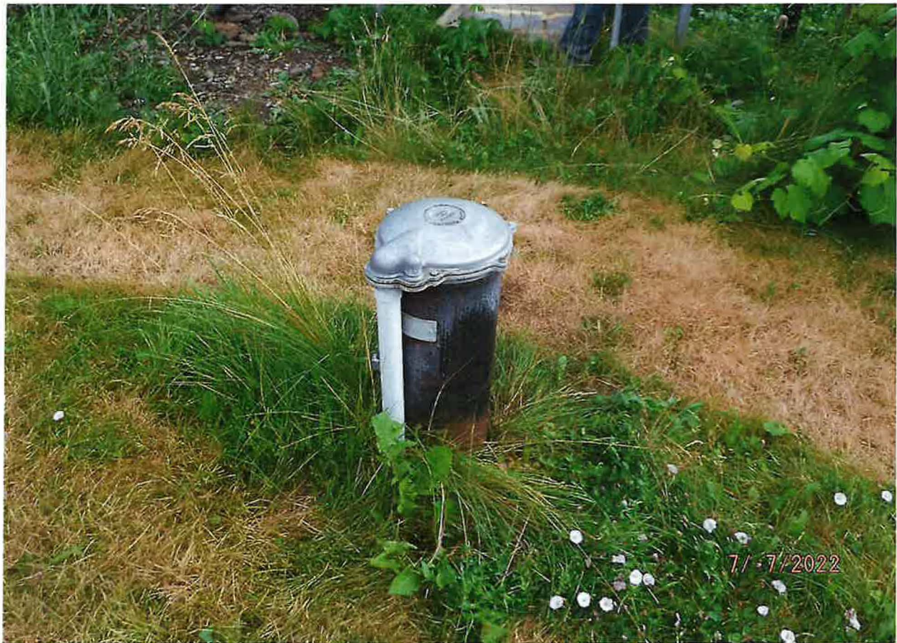
POD – GROUNDWATER WELL
