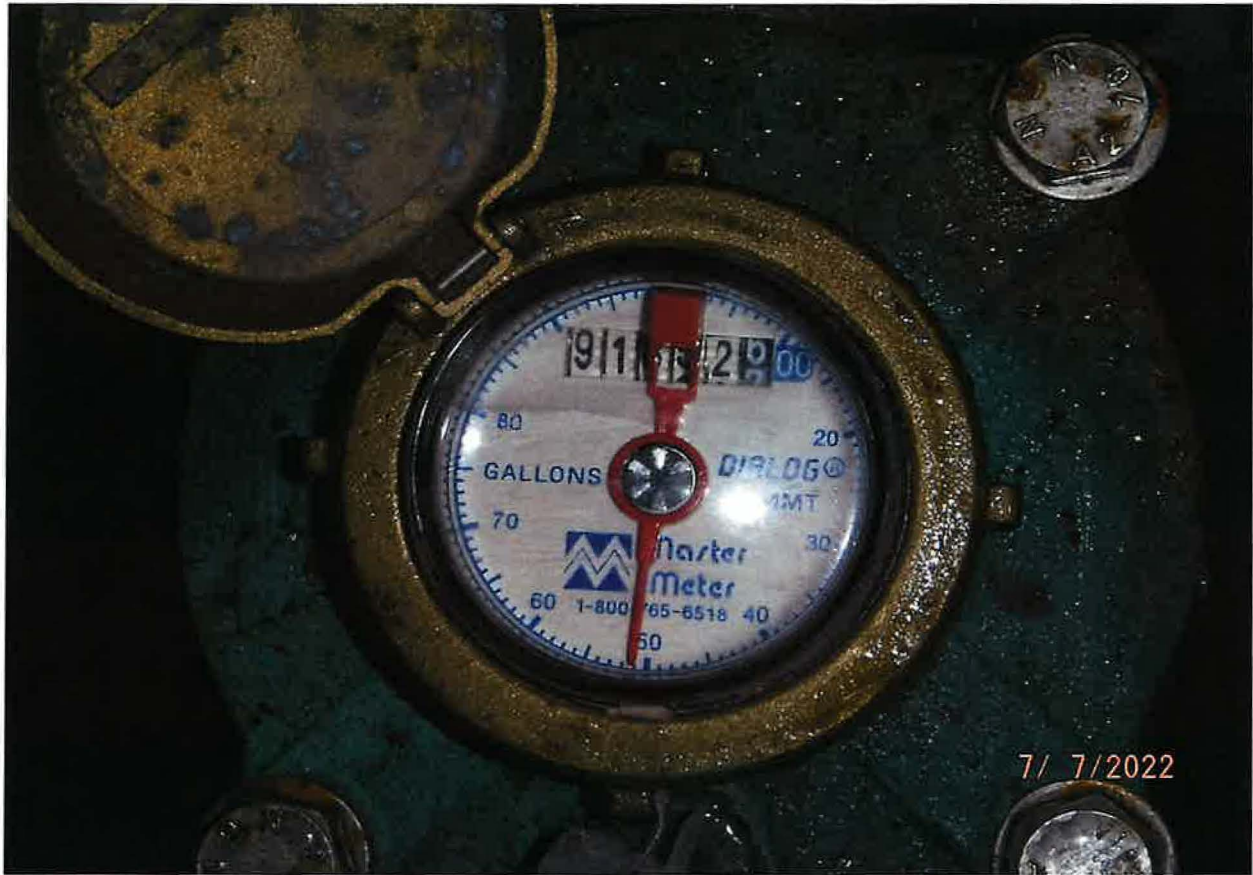
MASTER METER FLOWMETER INSTALLED ON SYSTEM
