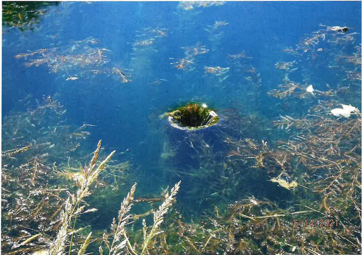
OVERFLOW DISCHARGE PIPE – RECREATION FLOW THROUGH DISCHARGES TO WETLAND AREA
