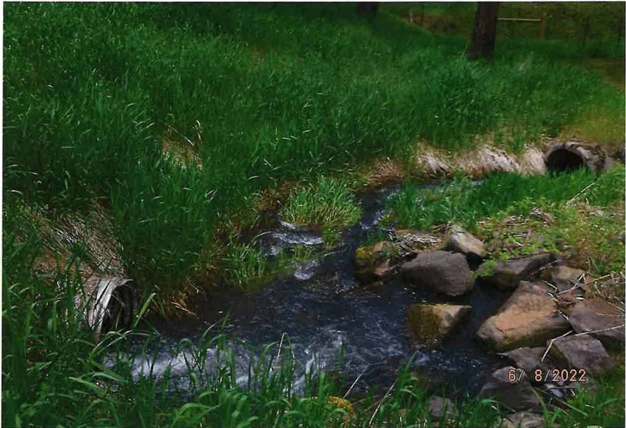
OVERFLOW PIPE ROUTING DOWNSTREAM AND THROUGH A ROAD CROSSING
