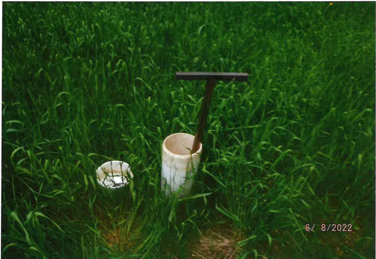
IRRIGATION FROM STORAGE MANUAL SHUTOFF VALVE, BURIED POLYPIPE TO FROST FREE HYDRANTS
