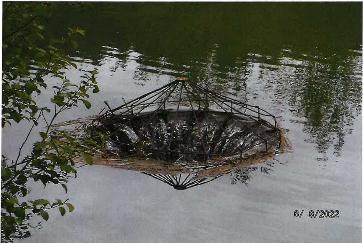
VERTICAL PIPE TO CULVERT OVERFLOW DEVICE LOCATED ON NORTH SIDE (DAM SIDE) OF POND
