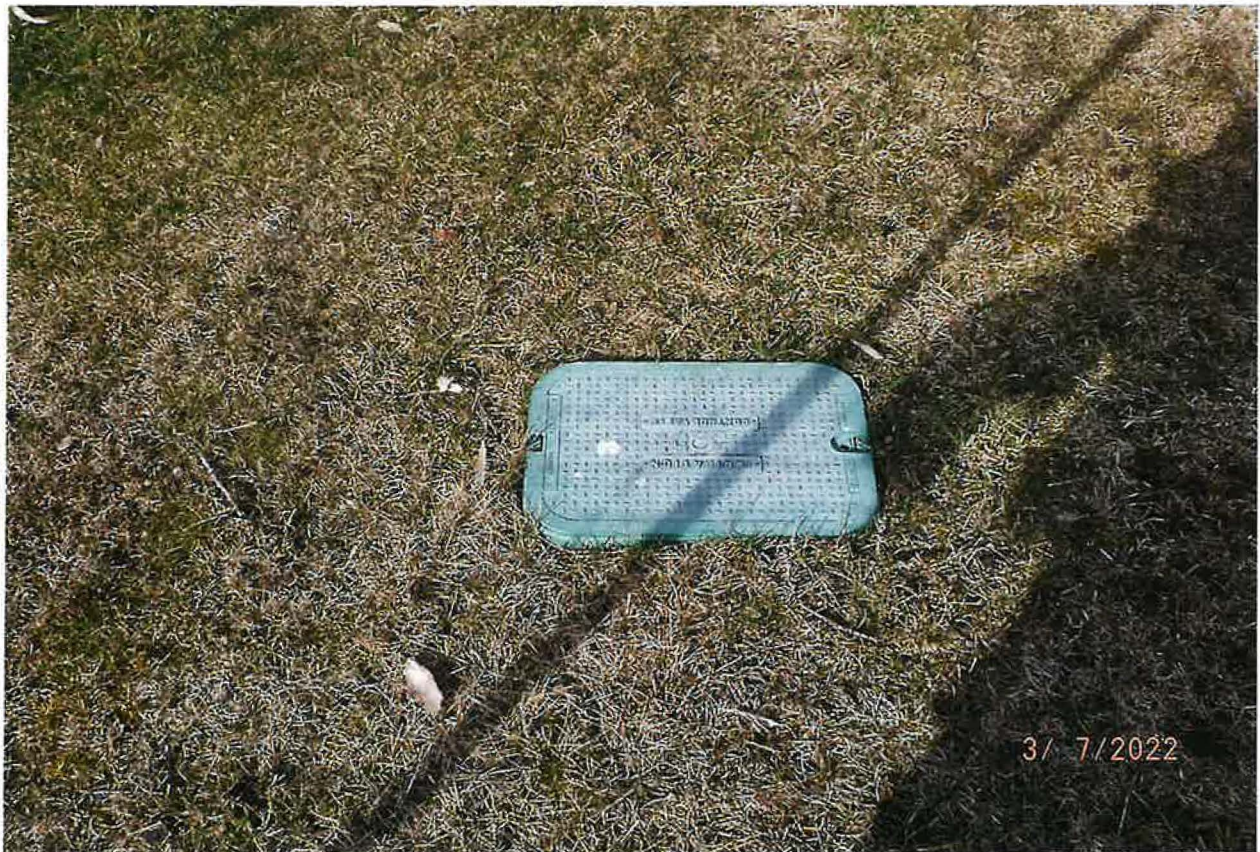
EXAMPLE – SPRINKLER ZONE BOX OFF YARD IRRIGATION TRUNK LINE
