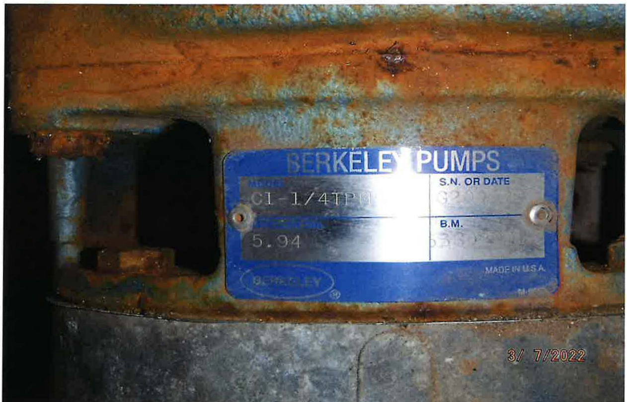
BOOSTER PUMP INSTALLED FOLLOWING INITIAL FIELD EXAM TO SUPPORT BIG WHEEL IRRIGATION USE
