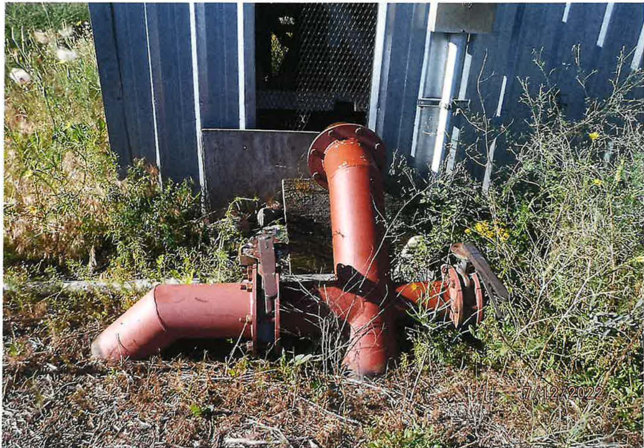
8 INCH MAIN LINE EXITING PUMP STATION ROUTING TO CENTER PIVOT, WITH OPTION TO ROUTE WATER Laterally EAST/WEST FOR HAND LINE OPERATIONS.
