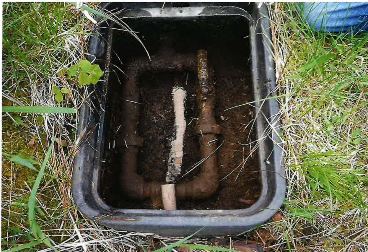
WATER SYSTEM MAIN SHUTOFF BALL VALVE – LOCATED AT POD ALONG SHORELINE
