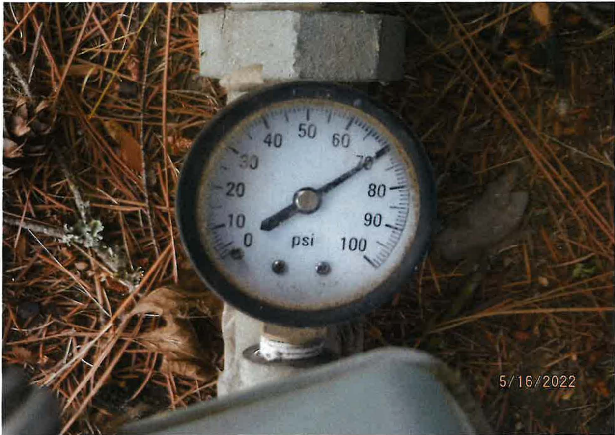
70 PSI HOLDING PRESSURE, OPERATING PRESSURE AT APPROX 60-70 PSI
