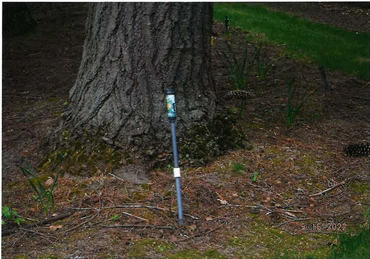
IRRIGATION POU - PRESSURIZED RAINBIRD SPRINKLERS, & ASSORTED HOSE TO SPRINKLER, AND LAWN STYLE IRRIGATION SYSTEMS IN PLACE RANDOM PER PARCEL BUT SERVED BY COMMON IRRIGATION MAIN PIPELINE TO IRRIGATION RISERS.
