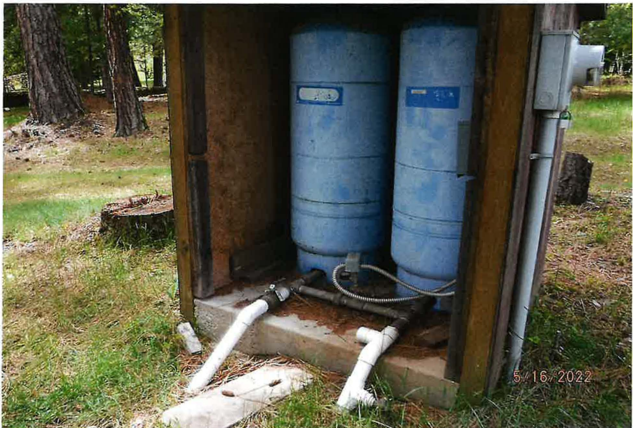
WATER SYSTEM POWER STATION – PUMP CONTROL HEAD LOCATED HERE – INFLOW ON LEFT, OUTFLOW TO IRRIGATION SYSTEM ON RIGHT; 2 EA PRESSURE TANKS INCORPORATED IN SYSTEM.
