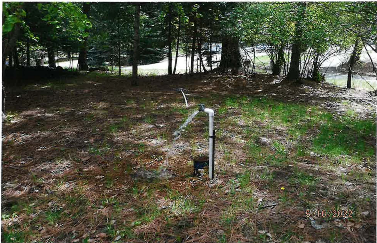
IRRIGATION POU – SERIES OF PVC RISER PIPES TO HOSE BIBS FOR IRRIGATION USE
