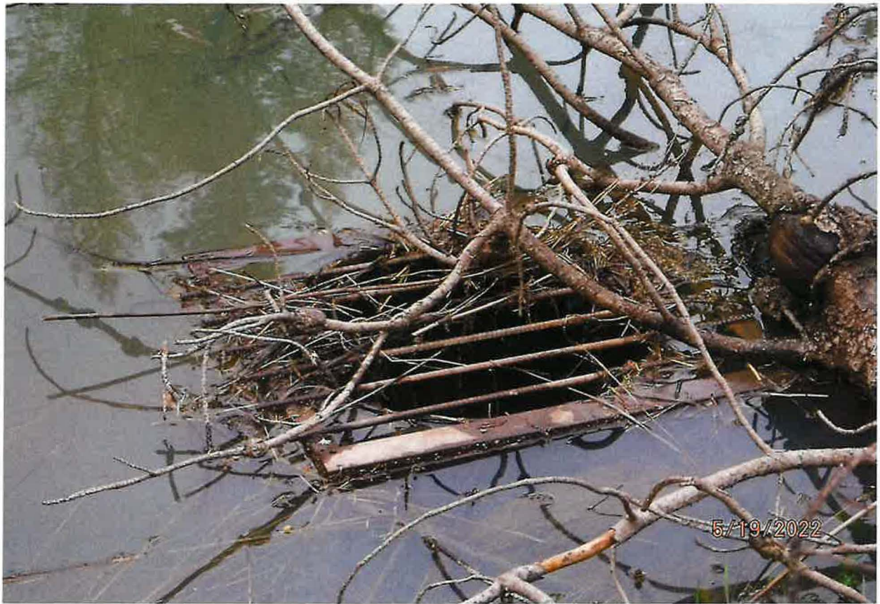
POND OVERFLOW DEVICE
