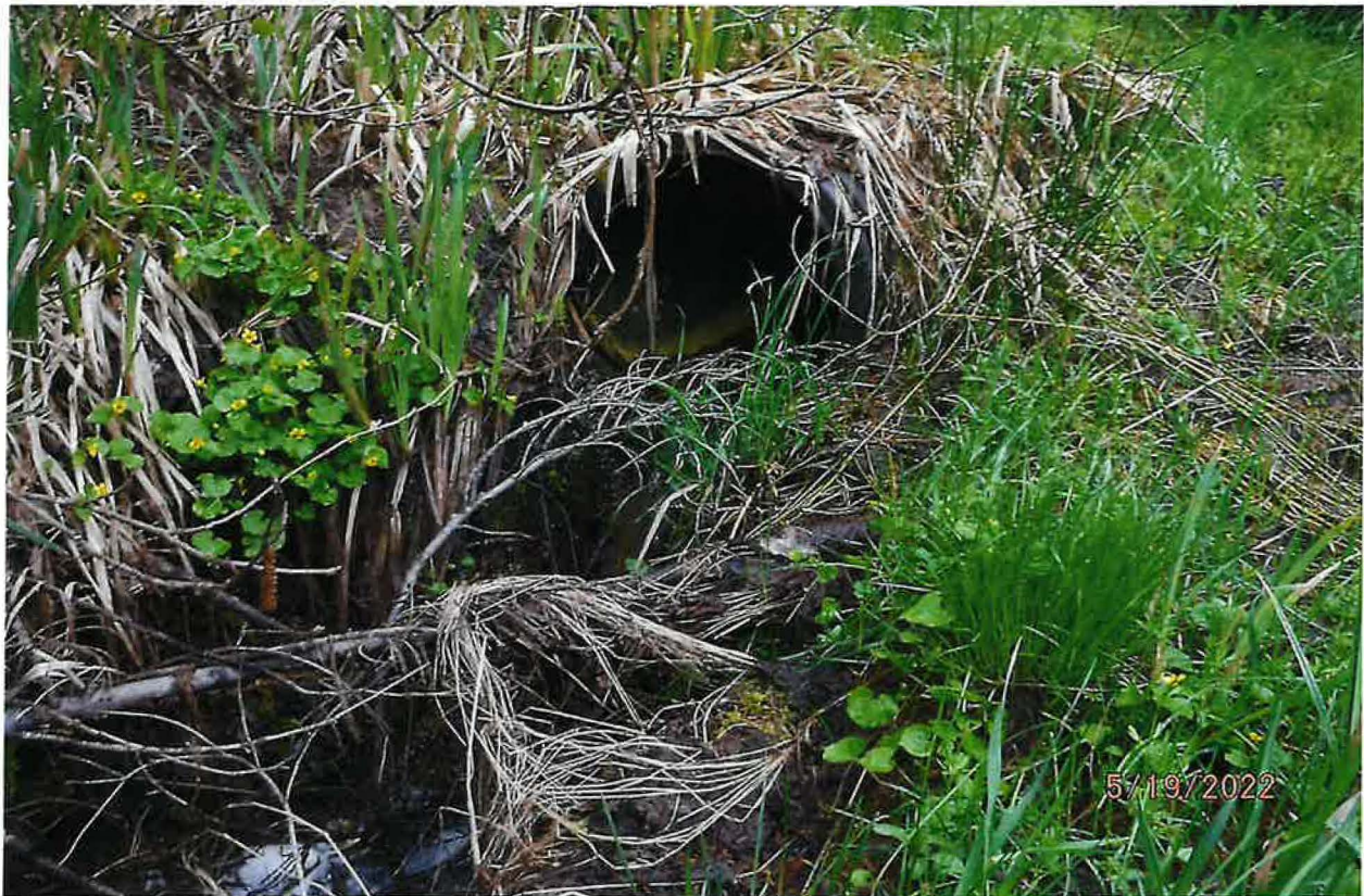
POND OVERFLOW DEVICE ROUTES WATER DOWNSTREAM
