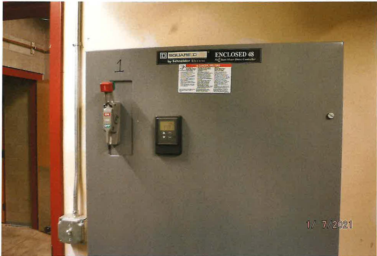
WELL 1 SYSTEM CONTROL PANEL – VFD 40 HP PUMP MOTOR INSTALLED IN WELL
