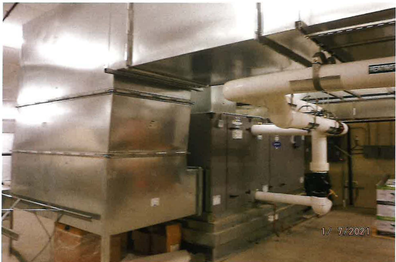
HEATING/COOLING SYSTEM DUCTING (UPSTAIRS IN KTEC FACILITY)
