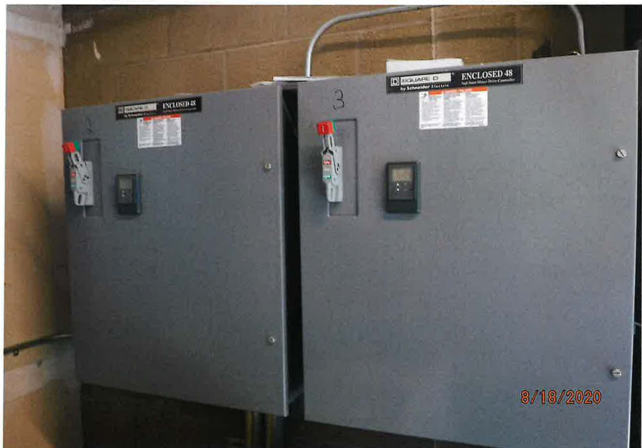
CONTROL PANELS FOR WELL(S) 2 AND 3
