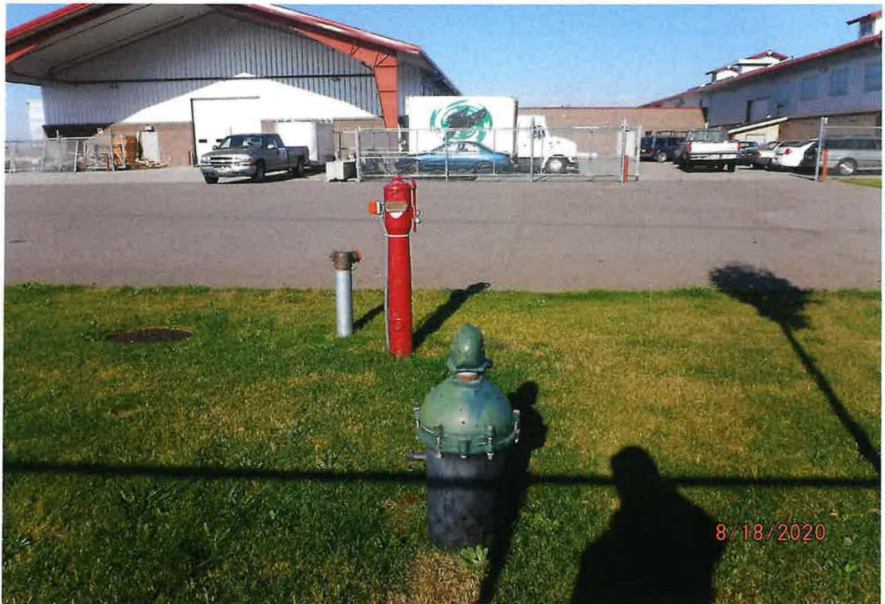
GROUNDWATER POD 2 OF 4 – WELL D-TAG D0060951, MIDDLE IN ROW OF 3 WELLS (PRODUCTION WELL)
