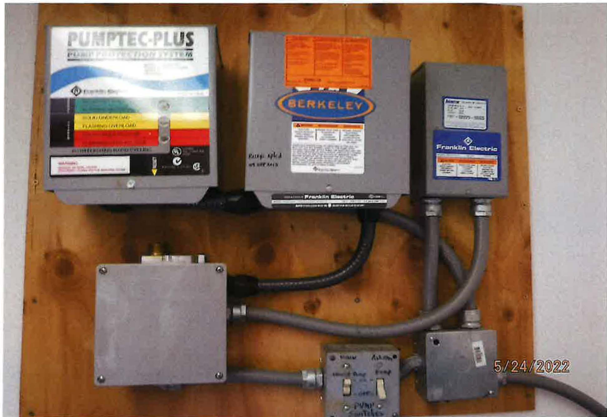
PUMP CONTROL PANEL IN SMALL PUMP STATION CO-LOCATED WITH WELL
