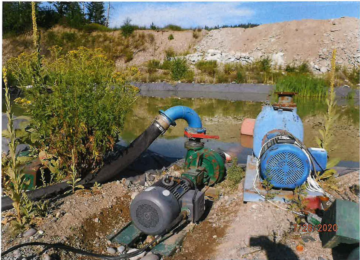
RECIRCULATION PUMP BACK TO INDUSTRIAL OPERATIONS
