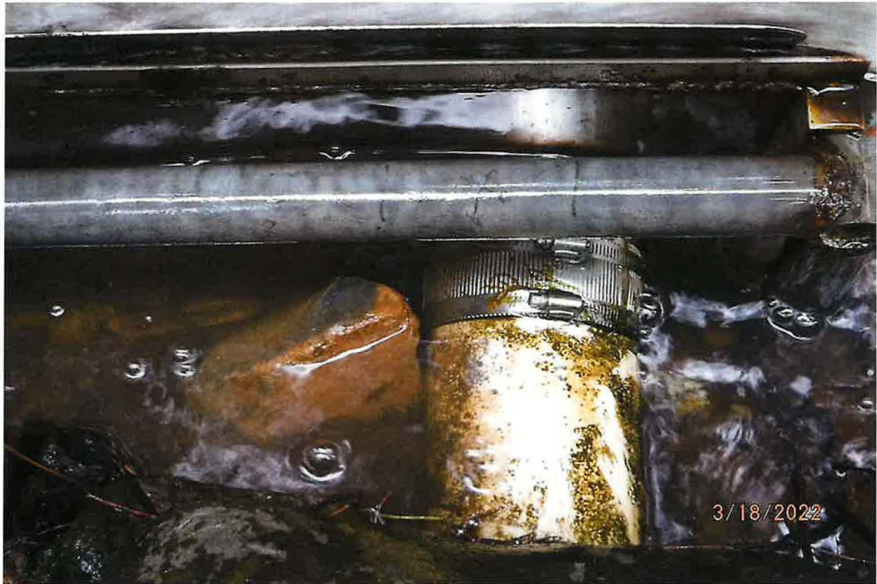
HYDRO POWER PENSTOCK – 4 INCH PVC PIPE WITH 181 FT OF HEAD
