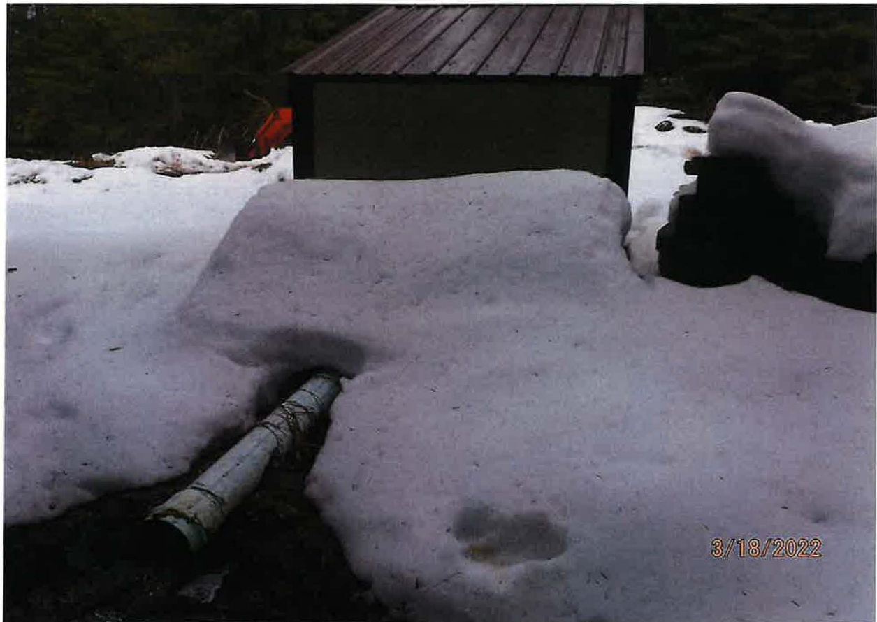
POWER POU – POWER STATION WITH OVERFLOW DISCHARGE 8 INCH STORM PIPE
