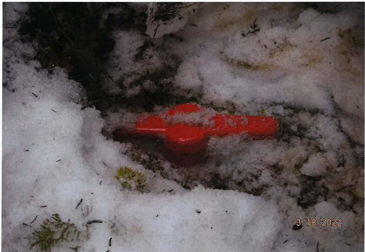
MANUAL SHUTOFF VALVE LOCATED AT PENSTOCK LOCATION ALONG SIDE STREAM
