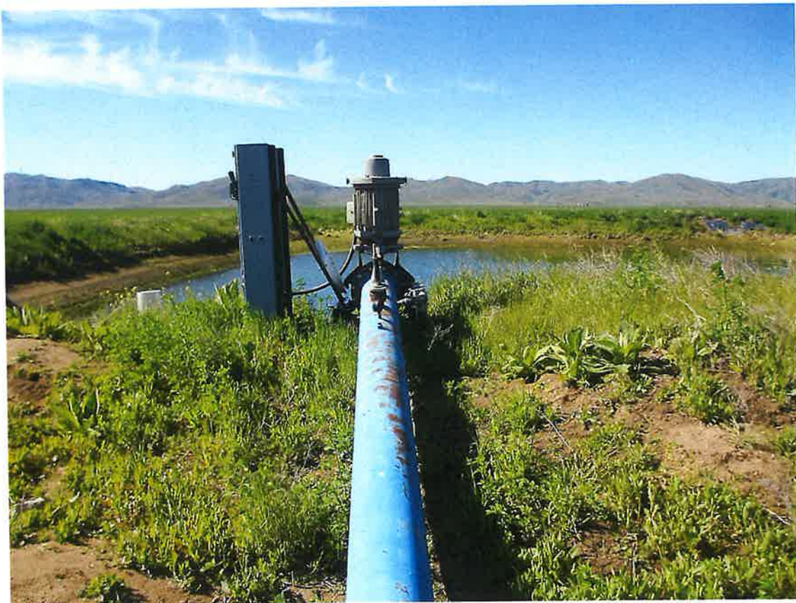
Pump and pipeline from pond to pivot
