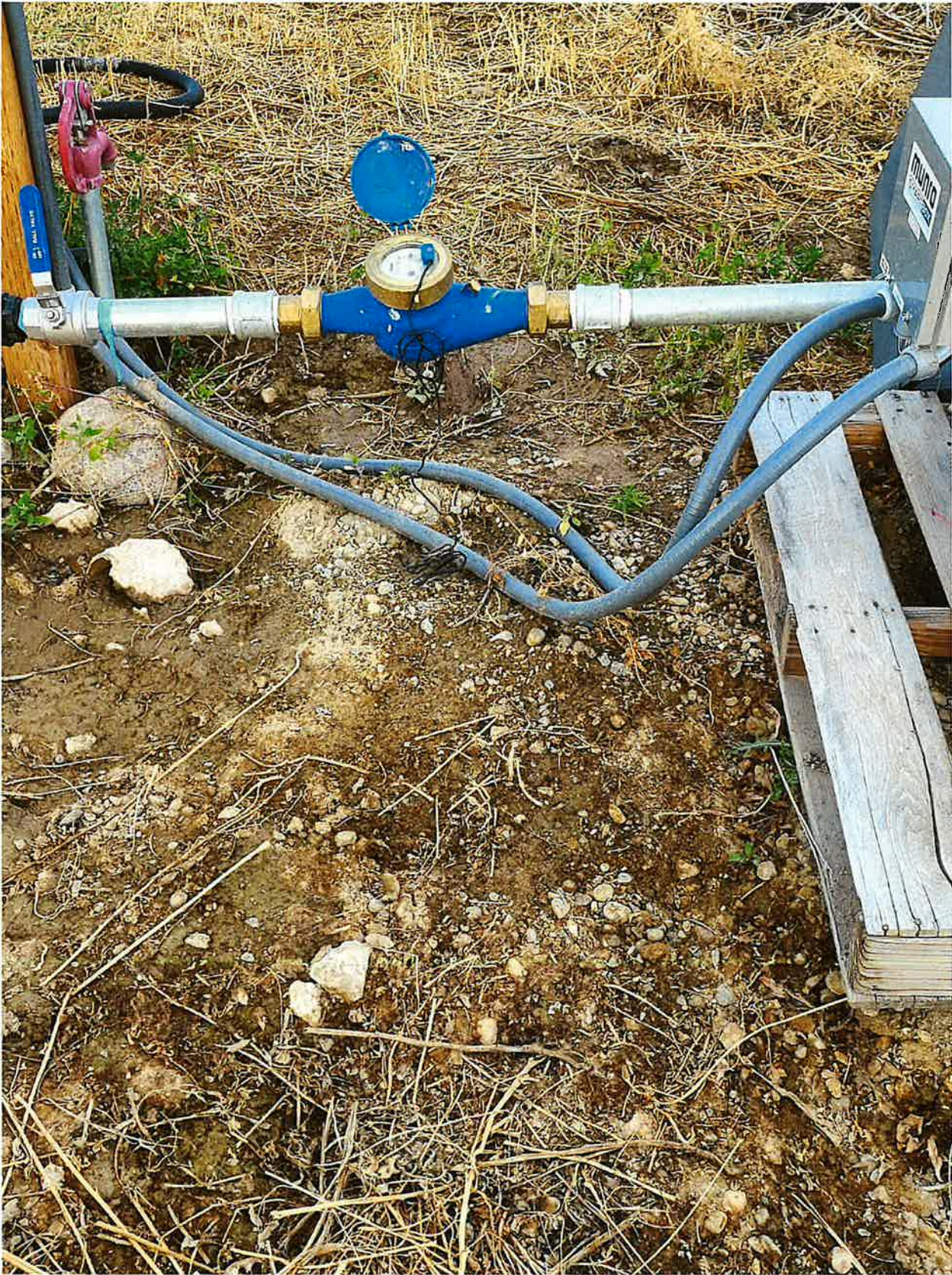
Water Flow Meter (to verify usage amounts)
