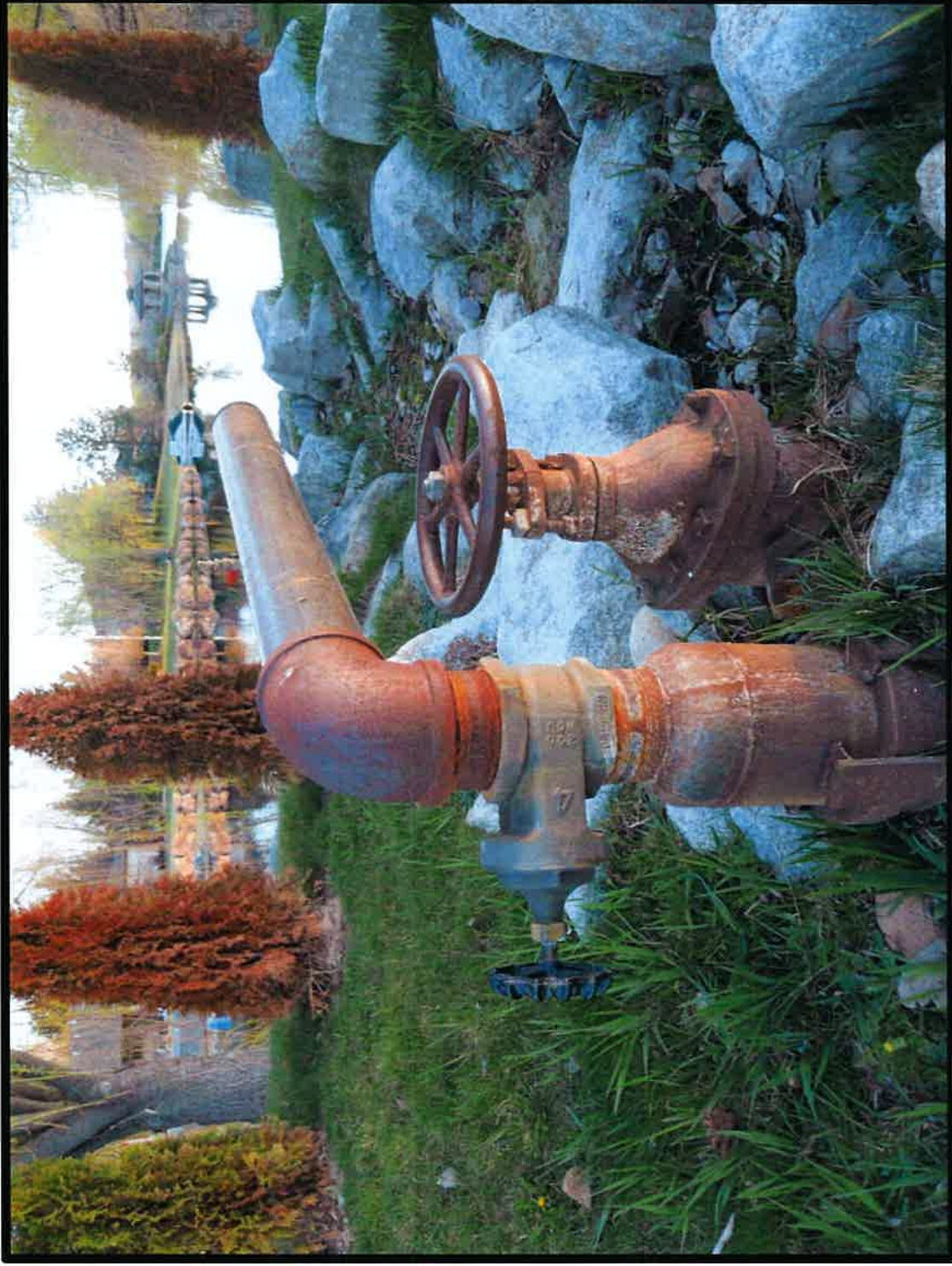
Artesian Well #3, Existing Water Feature, and Place of Use (Pond #1)
