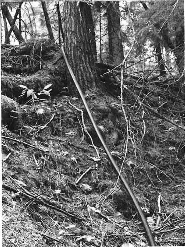
Poly pipe to carry water from Creek to Pressure tank.
