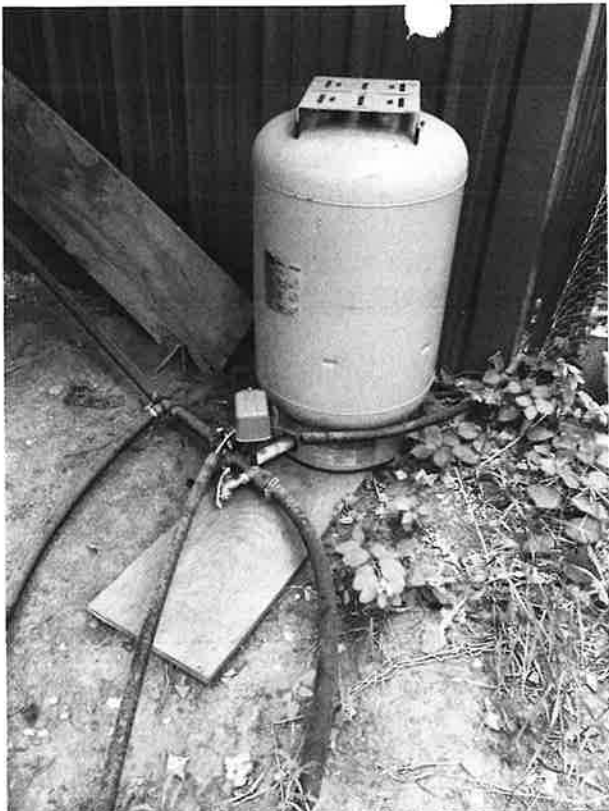
Pressure tank for Creek water
