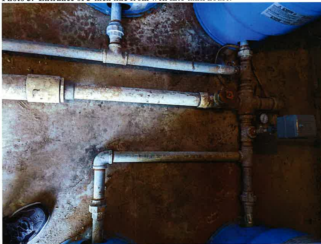
Photo 4. Manifolding of water line to five hydropneumatics tanks in tank house. Note pressure switch and gage.
