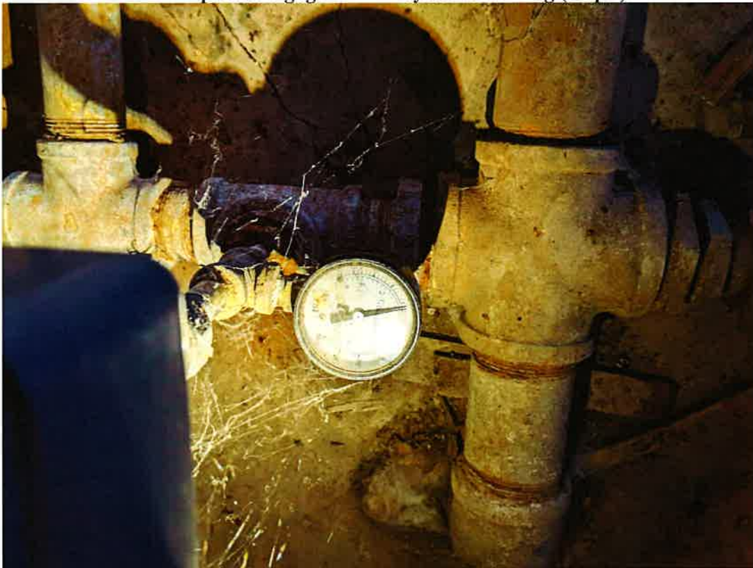
Photo 10. Tank house pressure gage with largest system running (42 psi).
