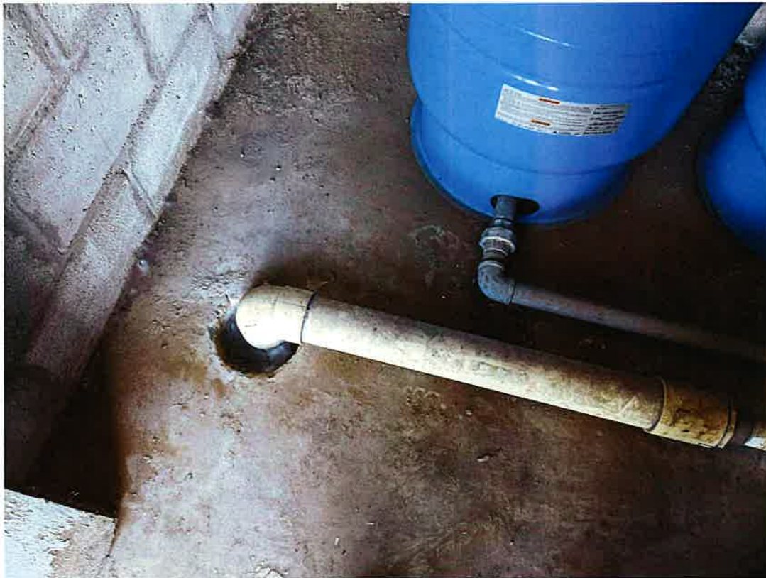
Photo 3. Entrance of 3-inch line from well into tank house.
