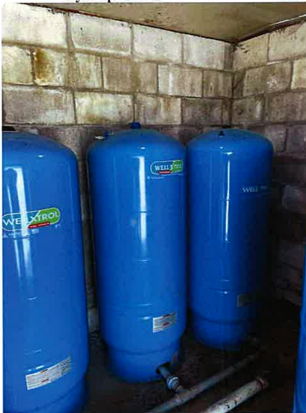
Photo 6. Three tanks on north side of tank building interior.
