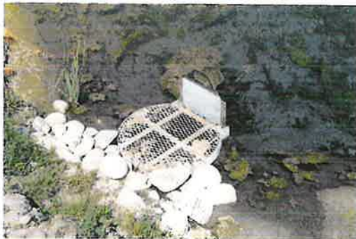
Slide gate in pond.
