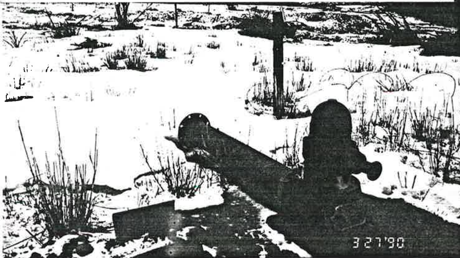
Close up of pump, pto hook up coupling in foreground, open discharge pipe pointing toward stream. Did NOT appear that there was any erosion from use (i.e. no gullies, washes or headcuts at stream bank).
