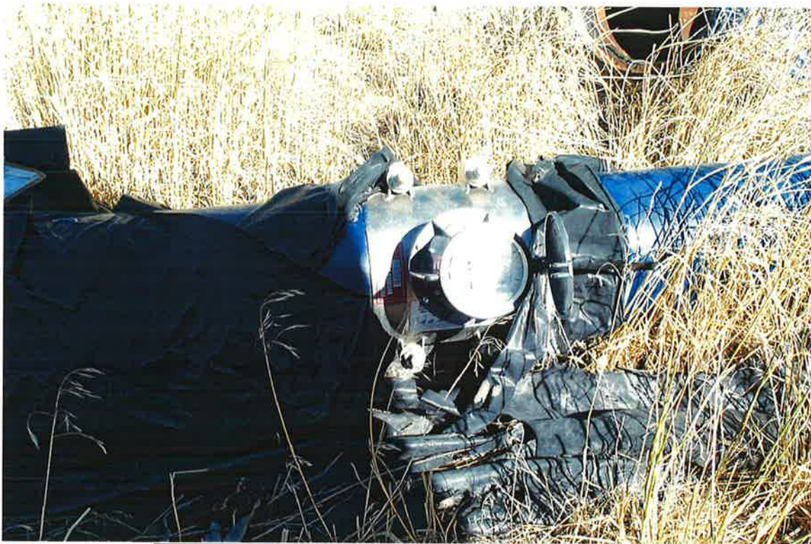
Flow Meter Laying On Ground Near Well – 37-7745A By J E Stanton 9-23-03
