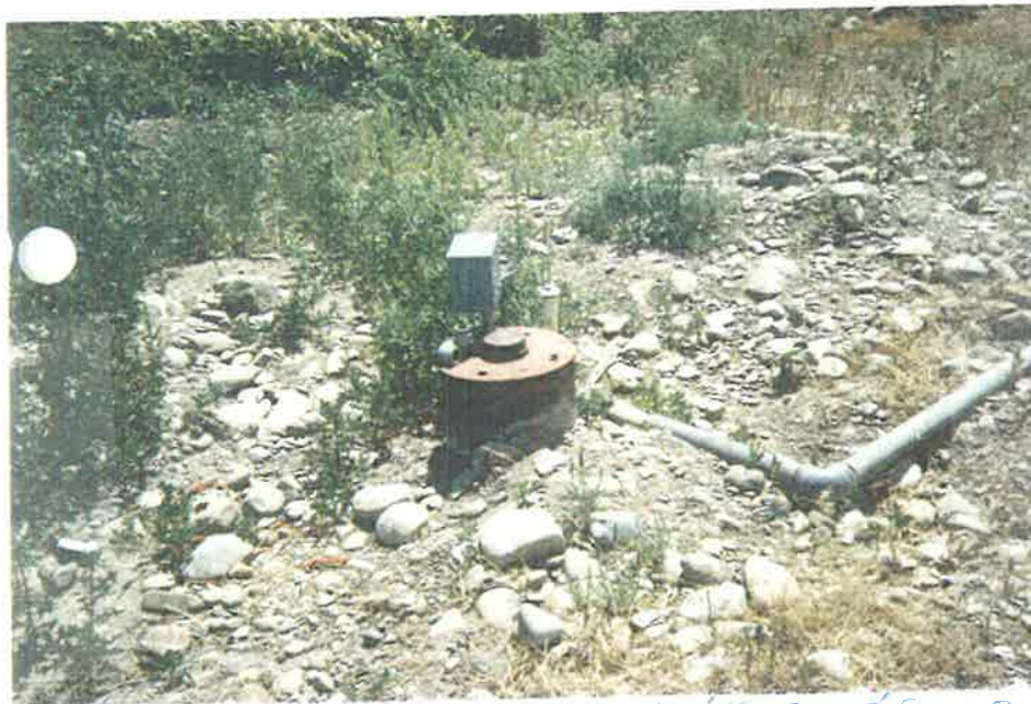
Submersible Well & motor & Pump.
