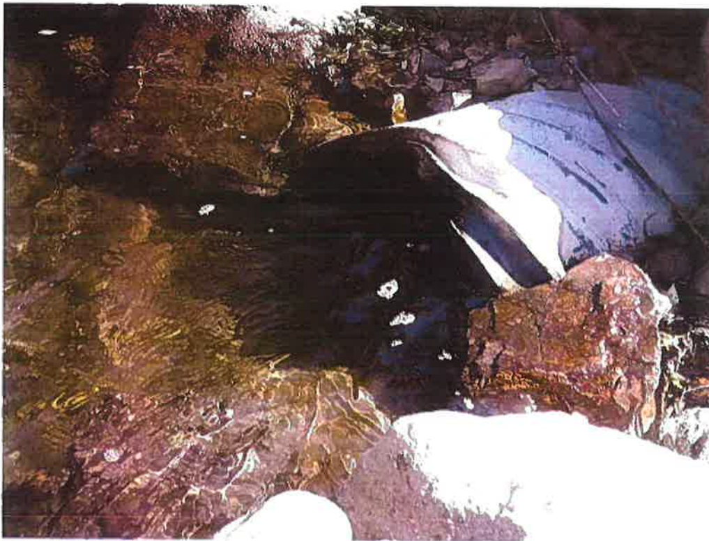
Creek end of 18" CMP. Note: sediment and lack of submerged state.
