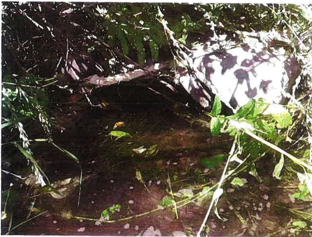
Pond end of 12" CMP. Note: flow is into the pipe and back toward the creek.
