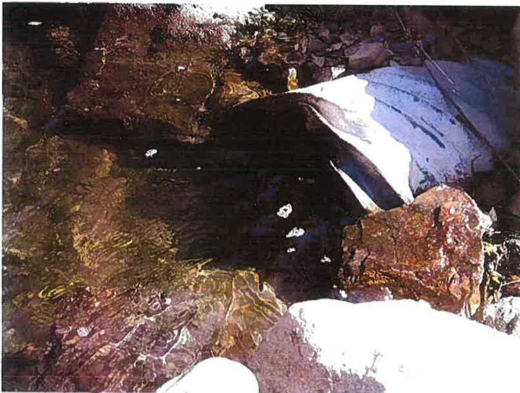
Creek end of 18" CMP. Note: sediment and lack of submerged state.
