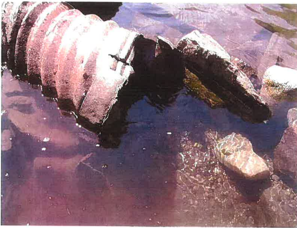
Creek end of 12" CMP. Note: water is flowing from the pipe into the creek.
