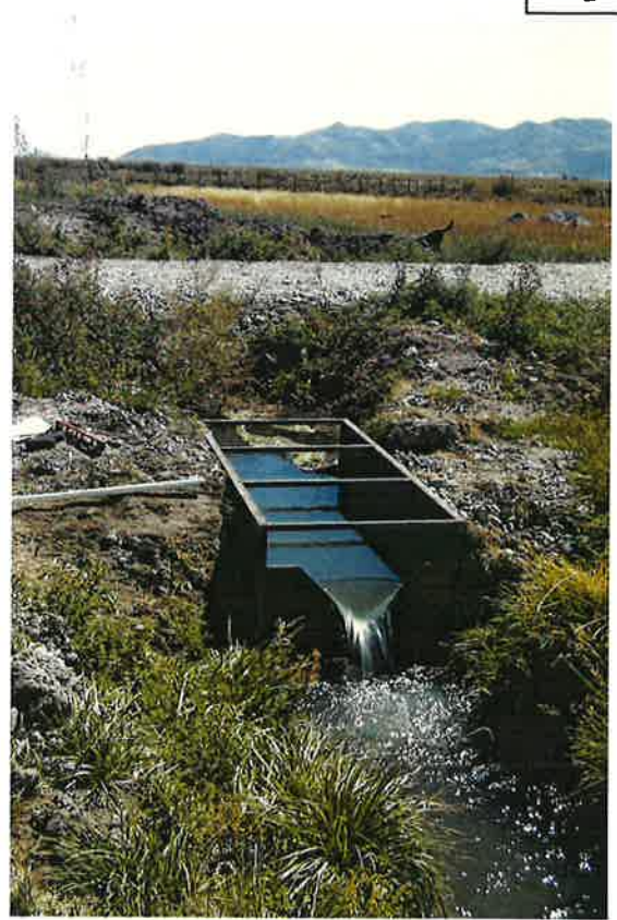
Smith – weir, measured at 0.82 cfs
