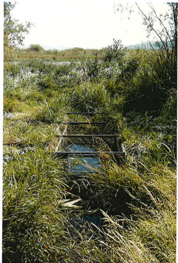
Dreyer weir – measured at 0.03 cfs
