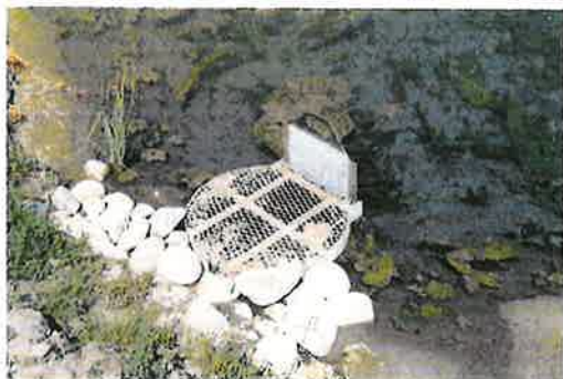
Slide gate in pond.
