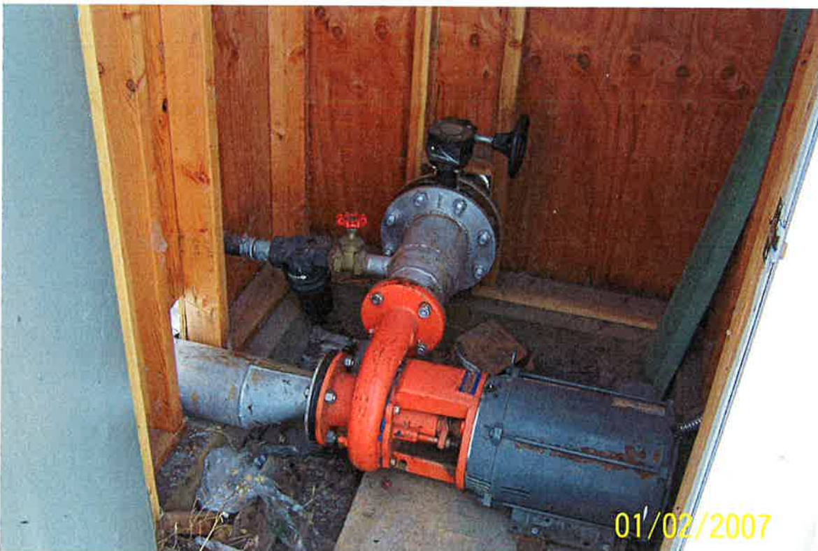
15 Hp Berkley pump Marathon motor 6" discharge 70 psi 2' lift
