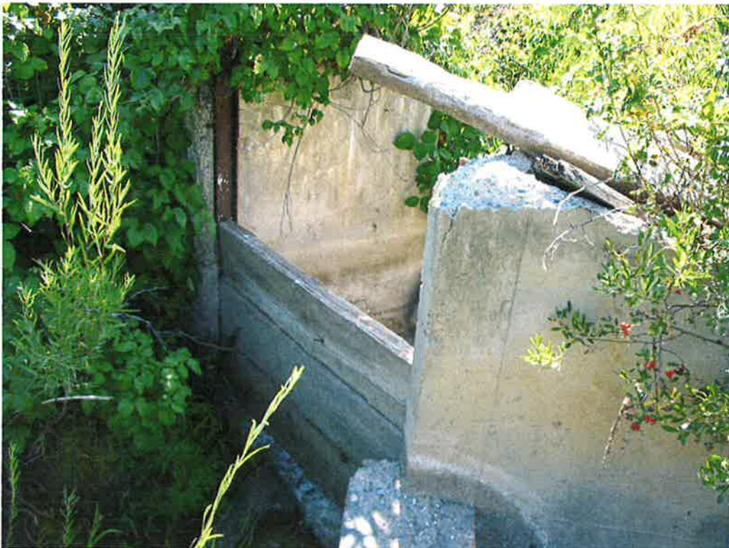
Photo of diversion taken during field exam by Lee Peterson.
