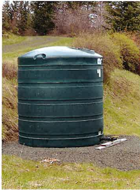
Figure 3: April 2017 image showing UIEF Portable Storage Tank 4 on constructed pad. Tank 4 is filled periodically from Fire Pond 8. Location of Storage Tank 4 is shown on attached POD / POU map.
