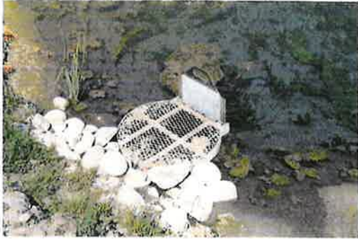
Slide gate in pond.
