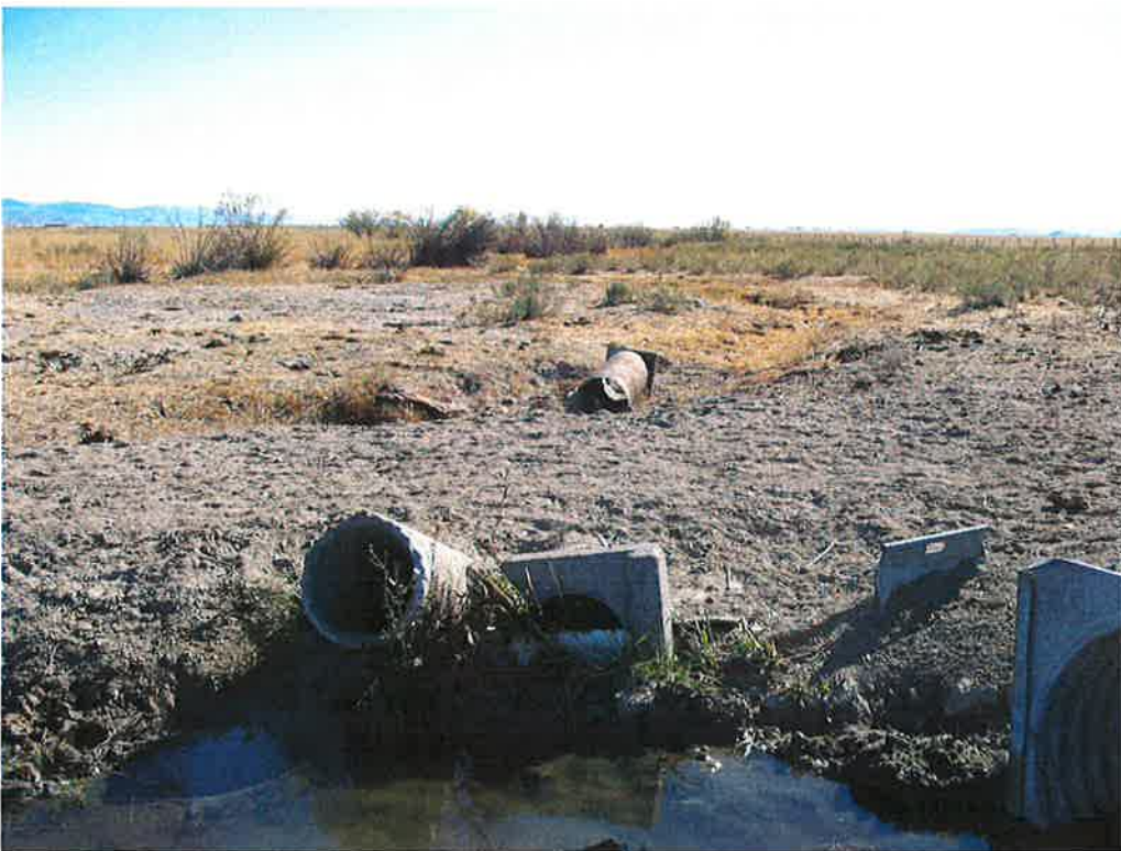
Photo of distribution system taken during field exam.
